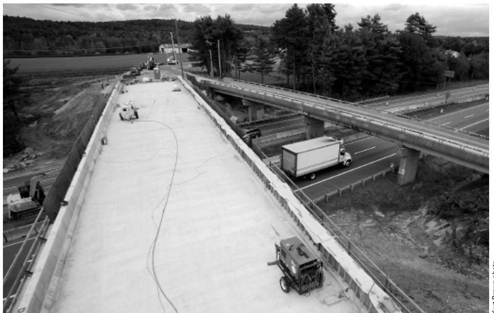
The completion of the new two-lane Mayall Road Bridge in New Gloucester puts the Turnpike Authority near the mid-point of its program to rehabilitate the highway's 176 aging bridges.
