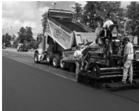
A paving crew on the Maine Turnpike. Timely maintenance of the paved highway saves money and improves safety and performance for customers.
