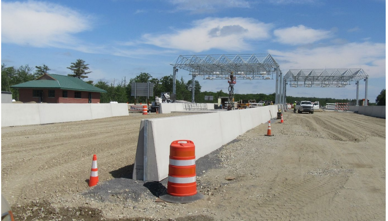
Space frame to the ORT tolling equipment recently installed
