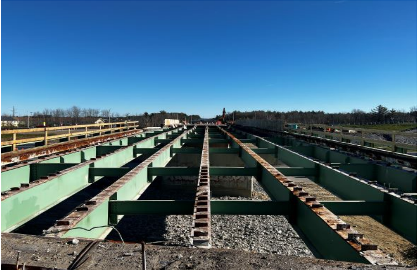
Looking east across the remains of the old Exit 45 bridge from the west approach.
