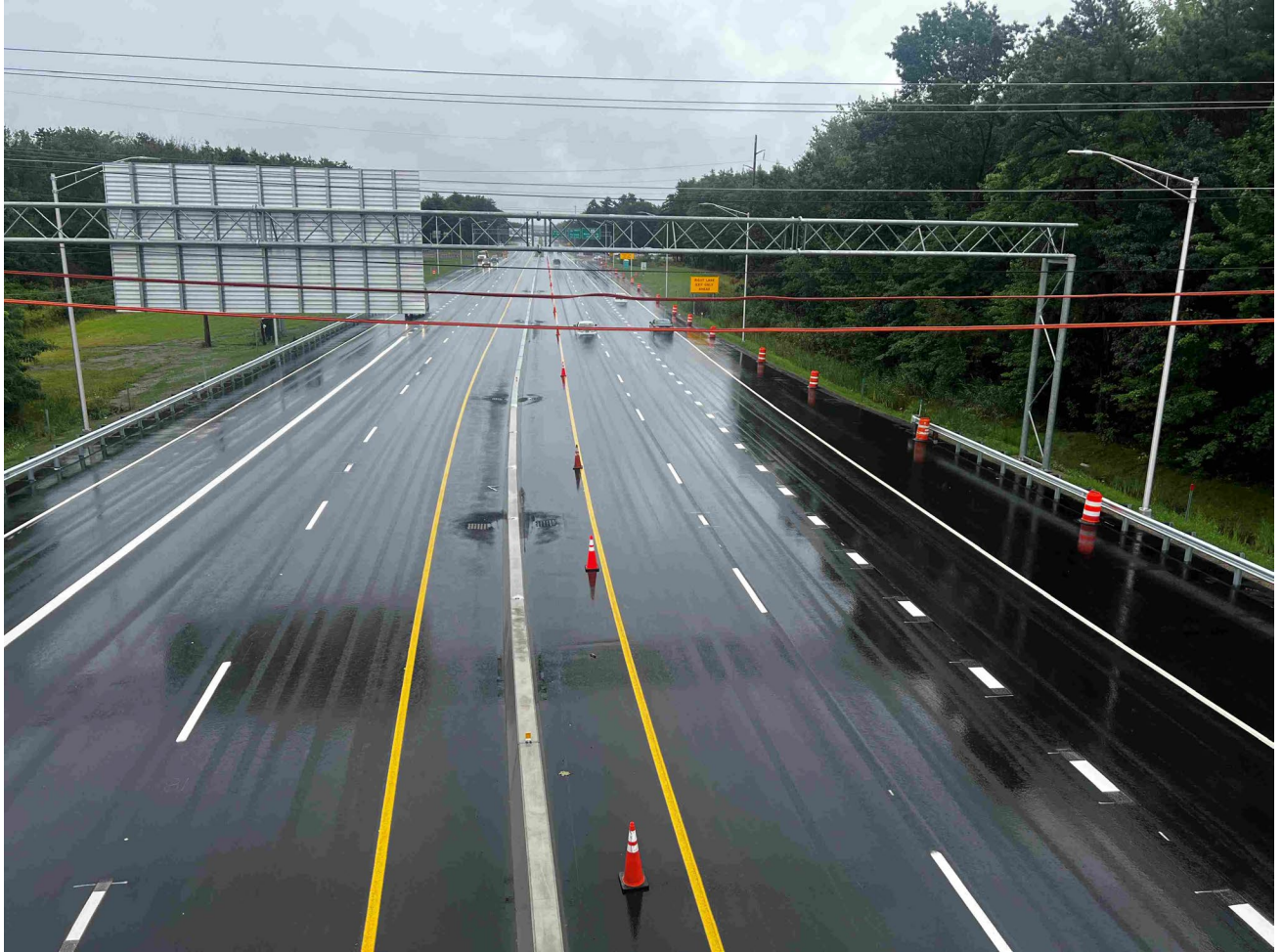
Looking east at the 703 connector with the new median barrier, surface paving, and final striping in place.
