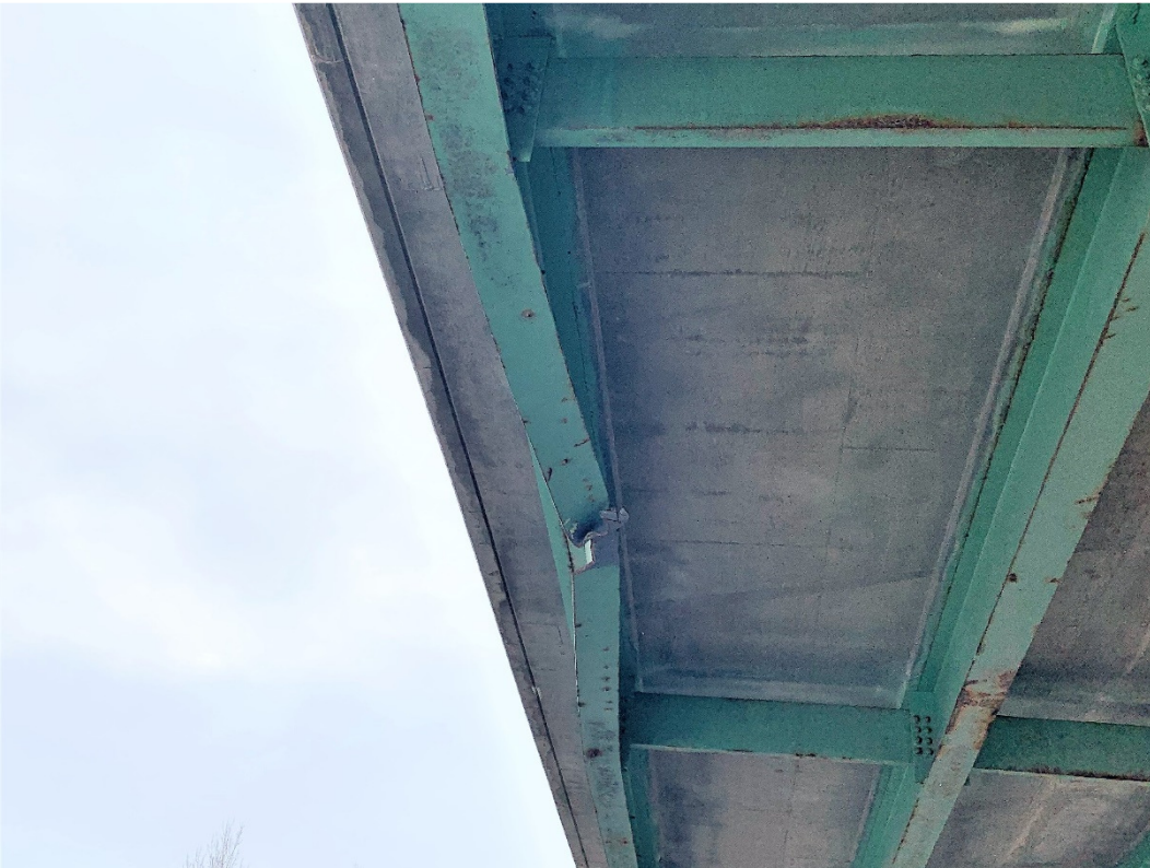
Figure 1 - Girder G1 Collision Damage (Looking East)
