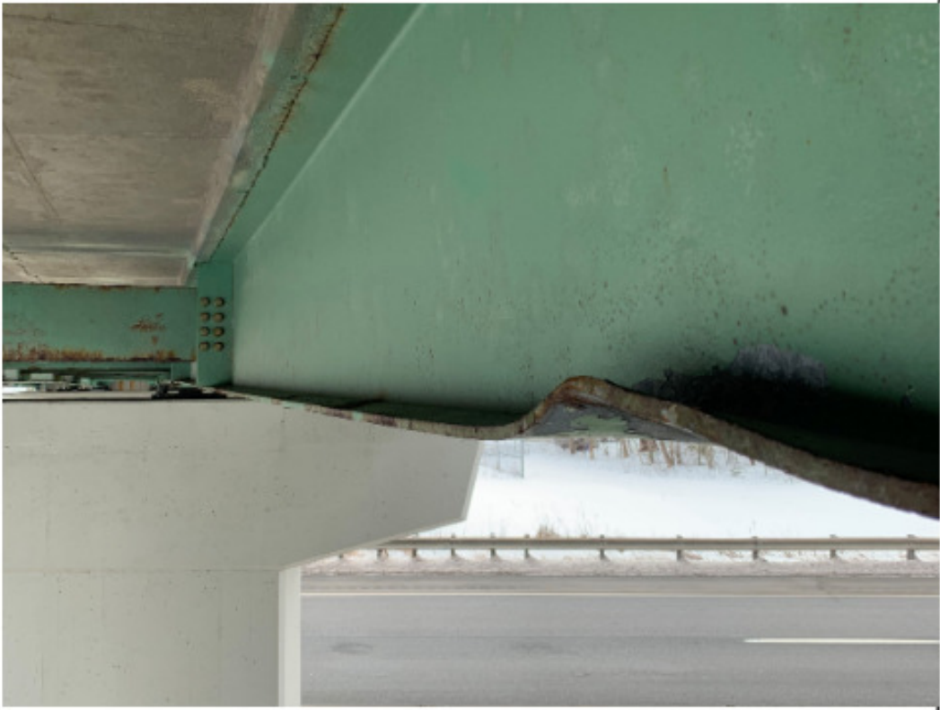
Photo 4 – Girder G3 Collision Damage – Bottom Flange Gouge and Deformation (Looking East)
