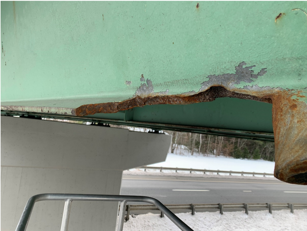
Photo 3 – Girder G1 Collision Damage – Bottom Flange Tear (Looking East)
