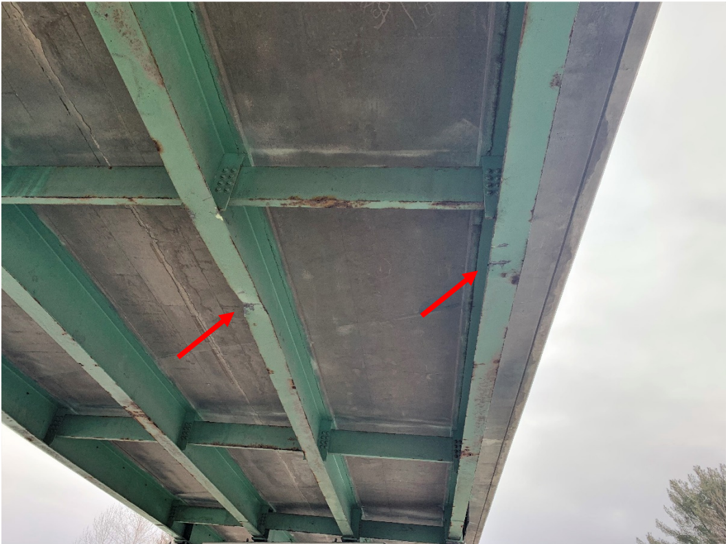
Photo 5 – Girder G2 & G4 Collision Damage (Looking East)
