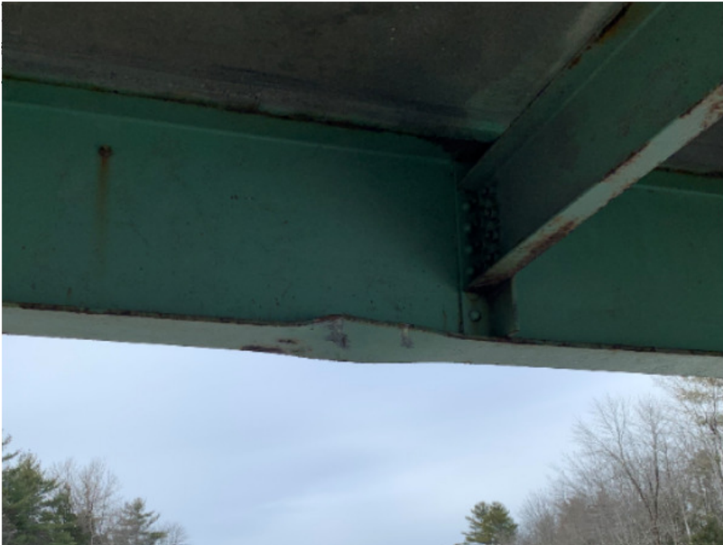
Photo 7 – Girder G4 Collision Damage – Bottom Flange Gouge (Looking South)
