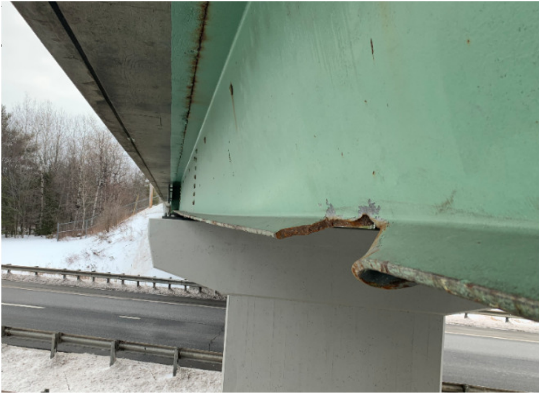
Photo 2 – Repair Area “A” G1 Bottom Flange Tear (Looking East)
