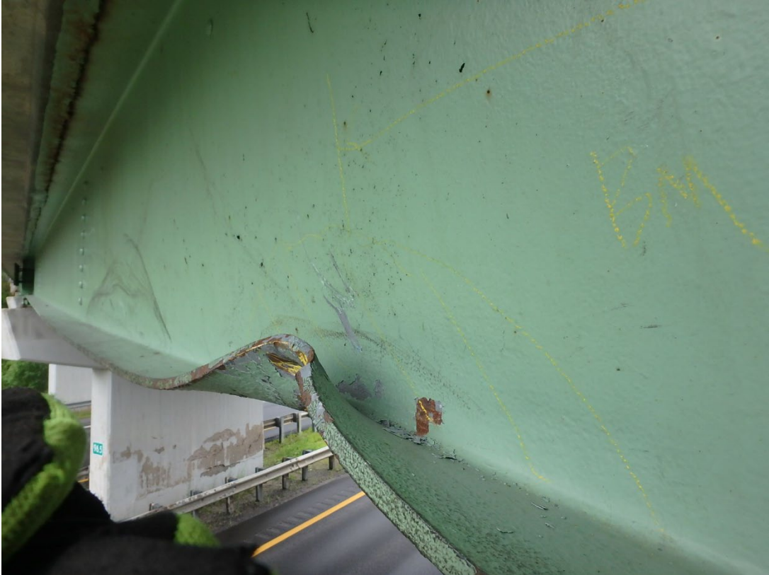
Girder G1: Collision Damage and bend with sweep, north face, looking south east
