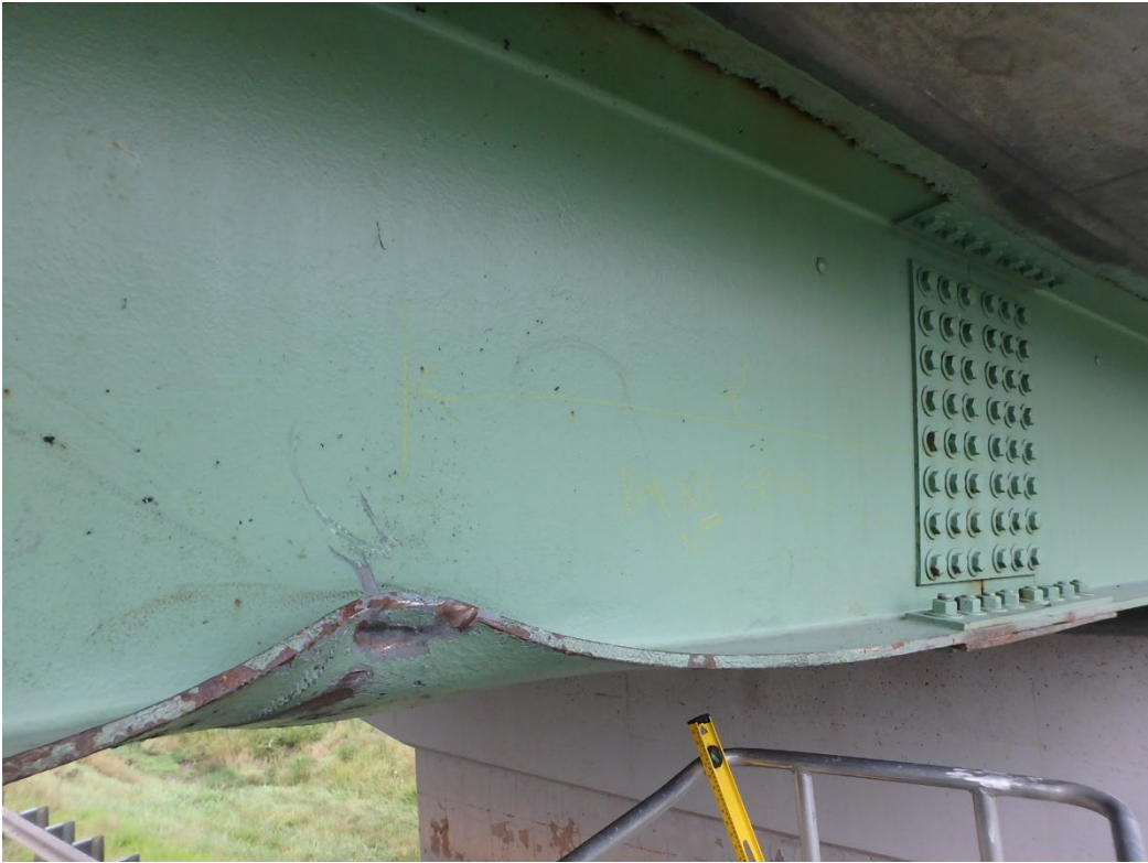
Girder G1: Collision damage, north face, looking south west
