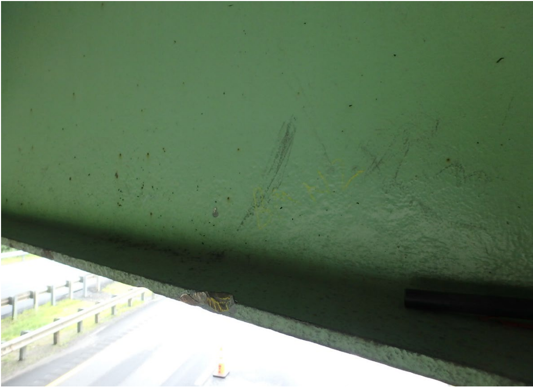
Girder G2: Bottom flange collision damage, looking south
