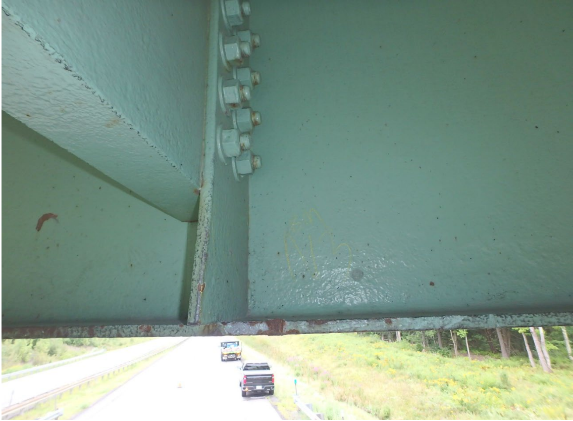
Girder G3: Bottom flange collision damage and bent stiffener, looking south
