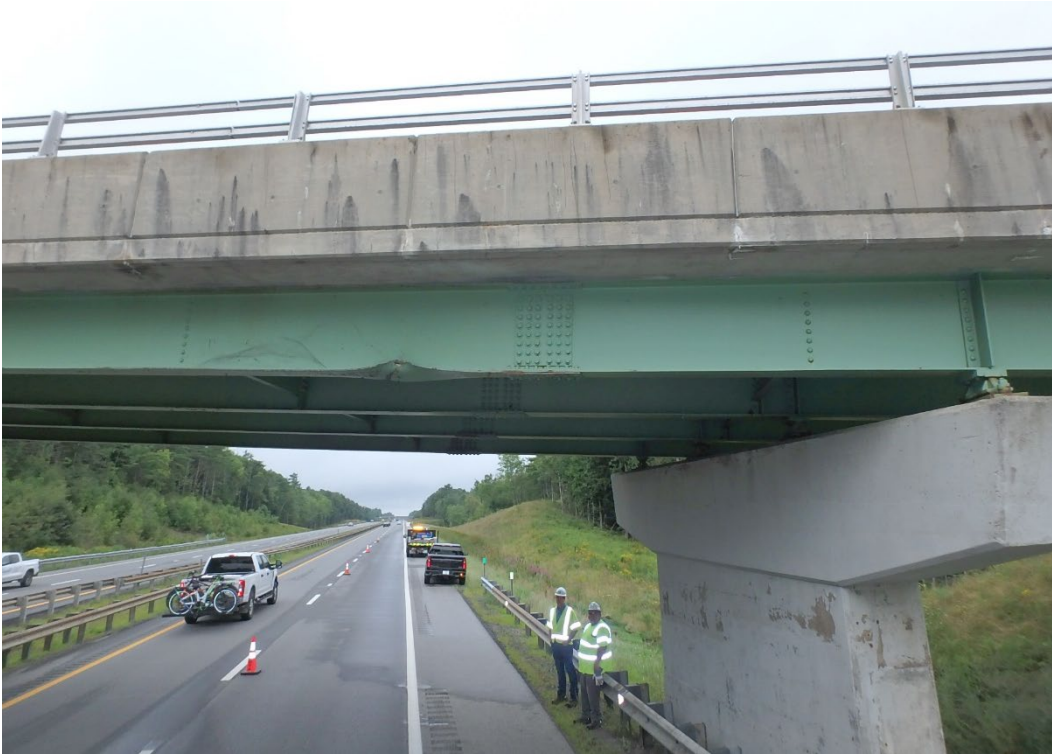
Stevenstown Road Bridge: Collision damage, elevation, looking south
