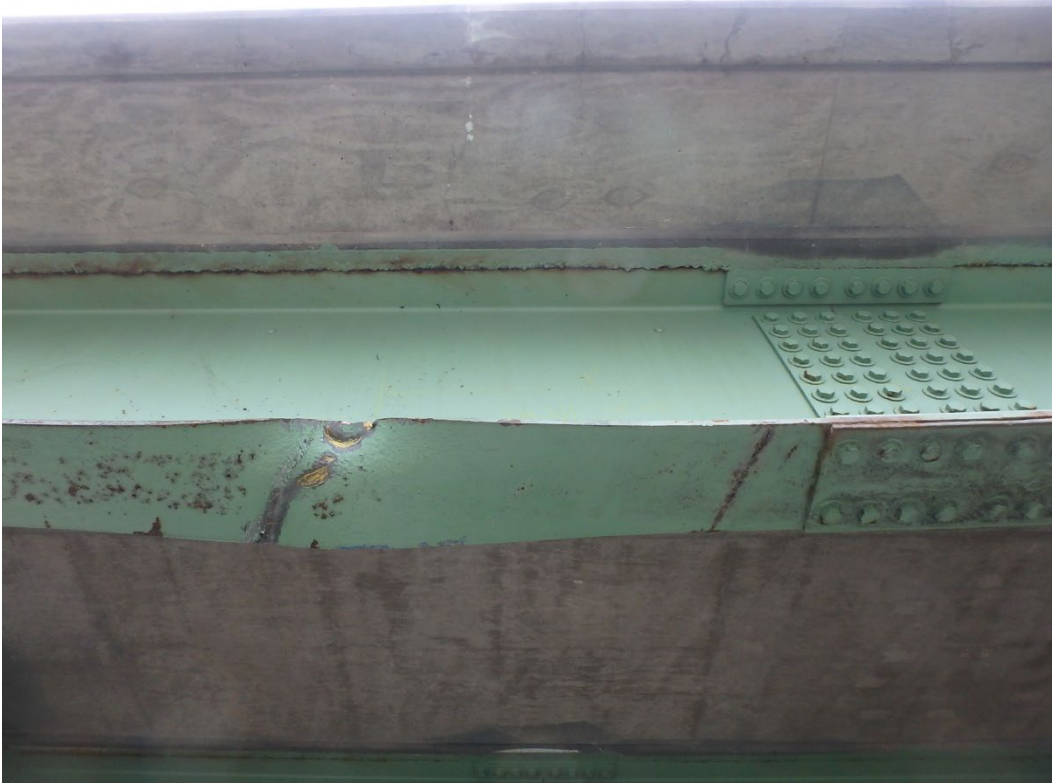
Girder G1: Collision damage, north face, looking up
