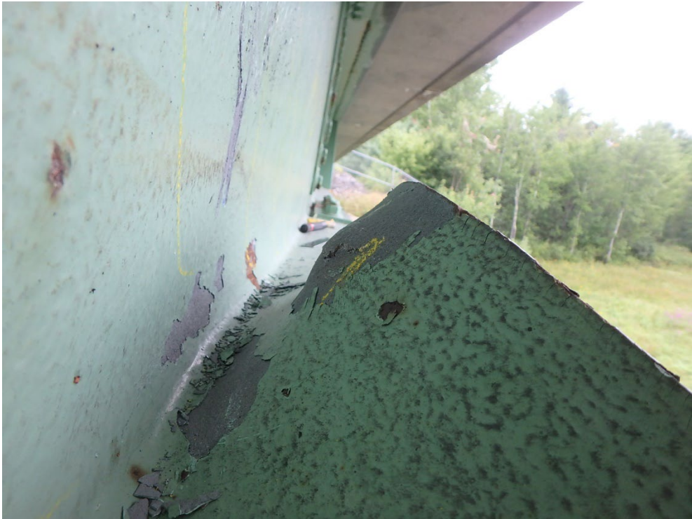
Girder G1: Collision damage and bend with sweep, crack in flange, looking west
