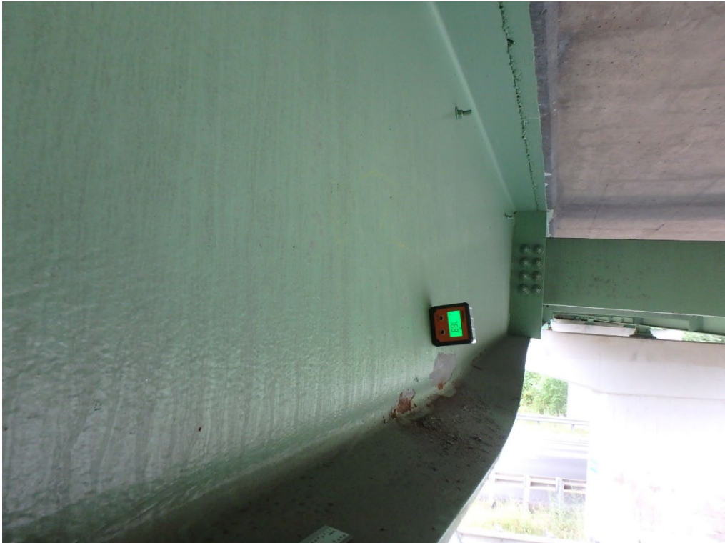
Girder G1: Flange distortion and web sweep, south face, looking east
