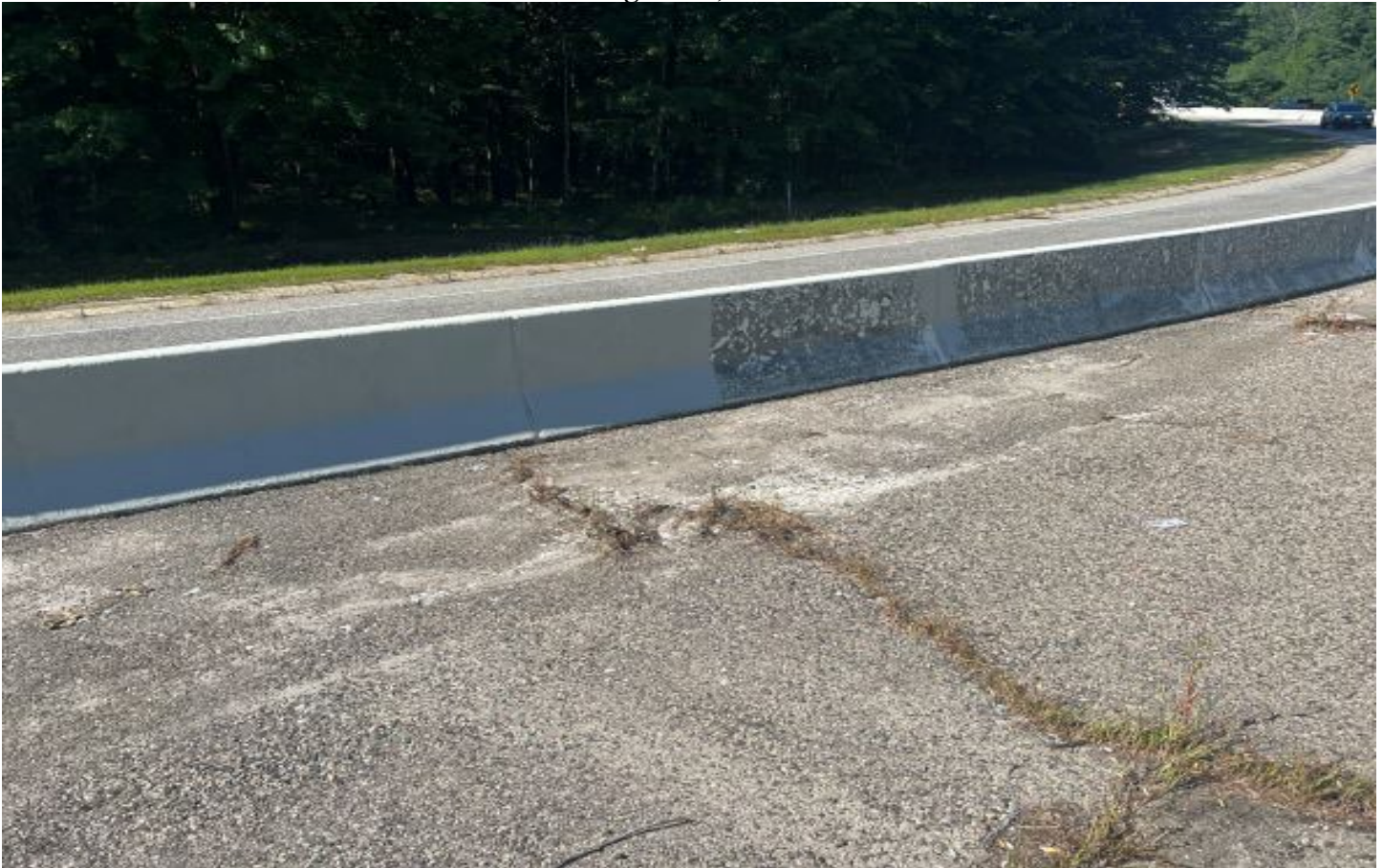
Exit 36 southbound ramp barrier showing a before and after for the pigmented coating repairs.
