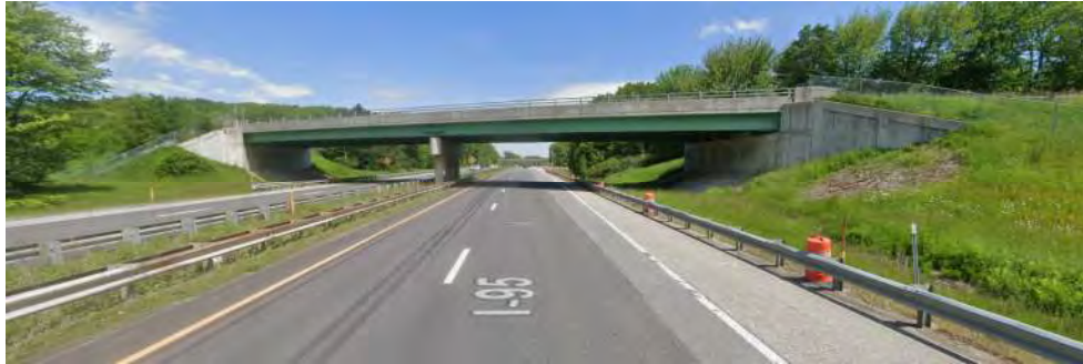
Photo 1: I-95 NB South of Exit 47 Off Ramp (2019)
