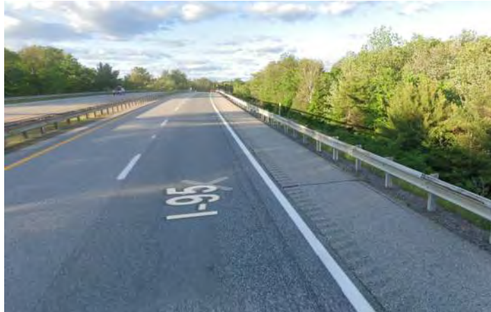
Photo 2: I-95 NB Just South of Exit 75 (2019)
