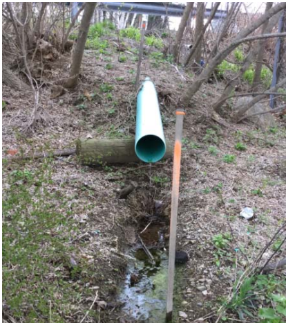
This outfall, though in poor condition because it is cantilevered, provides a good opportunity for a clean catch of its discharge.
