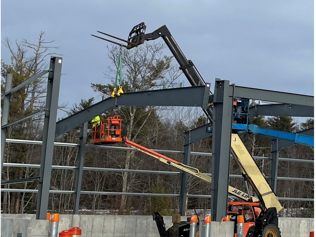
A Construx crew is hanging steel for the new 6-bay garage in York
