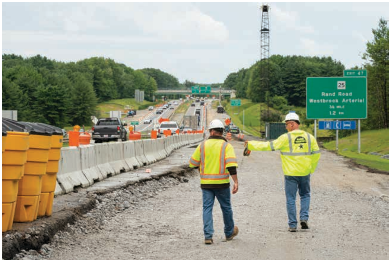
MTA staff reviewing traffic control measures at the Stroudwater River Bridge, July 2019.
