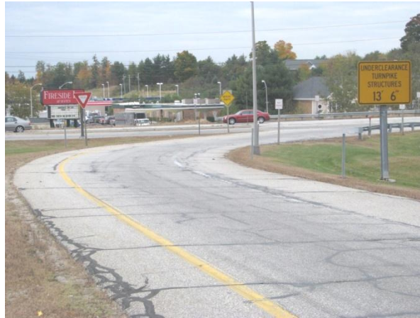
Figure 6 - Right slip lane onto on ramps from Route 202/4/100 southbound (Note significant crack sealing and large cracks)
