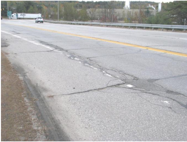
Figure 4 – Looking at Route 202/4/100 intersection from Turnpike approach (Note significant crack sealing, large cracks and patched pothole)
