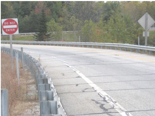
Figure 2 – Northbound off-ramp towards traffic (Note crack sealing)
