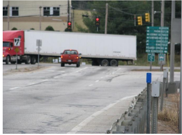
Figure 5 - Turnpike approach to the Route 202/4/100 intersection (Note extent of cracking)
