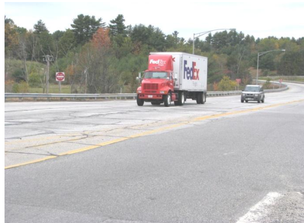
Figure 3 –NB & SB off-ramps approaching Route 202/4/100 intersection (Note crack sealing for Turnpike exiting lanes and overlay for entering lanes)
