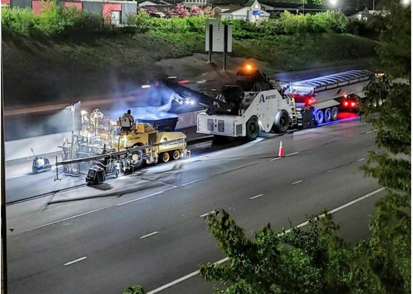
Looking south from Brighton Ave., the paving train is placing surface in Lane 1.
