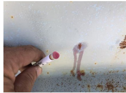
Figure 4: Lead based paint on Structure
