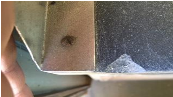
Figure 3: Asbestos containing Lab Tops
