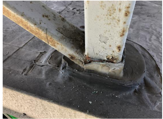
Figure 2: Roof Support beams Asbestos caulking
