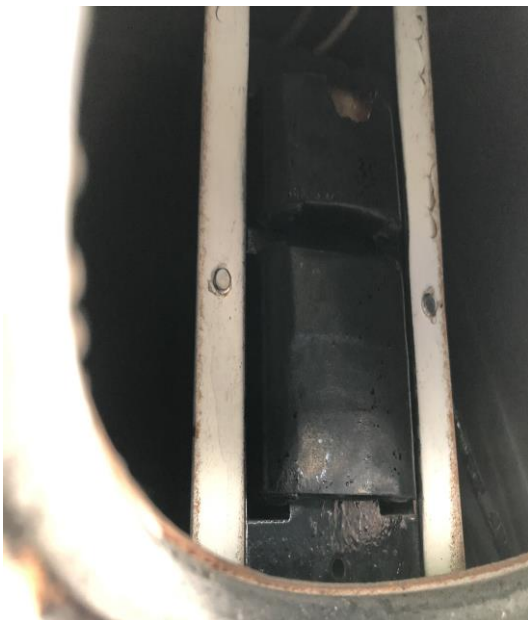
Figure 3: Presumed PCB ballast in old Lights
