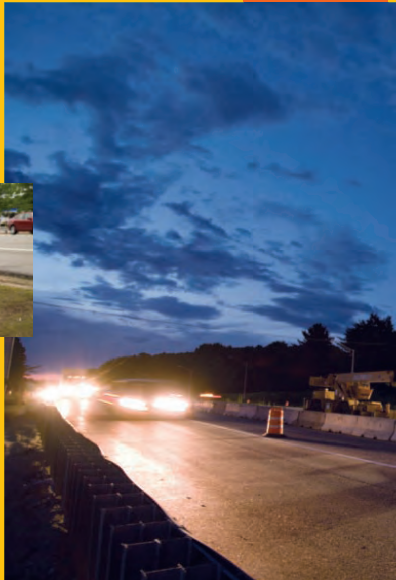
The Maine Turnpike fast-tracked construction on the Congress Street Bridge in Portland. The bridge that carries 14,000 vehicles a day, was rebuilt in just nine months by Technical Construction of Turner, Maine.
