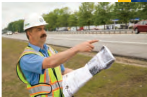
Project Manager Scott Warchol is one of several staff members who oversee quality assurance on Maine Turnpike projects.
