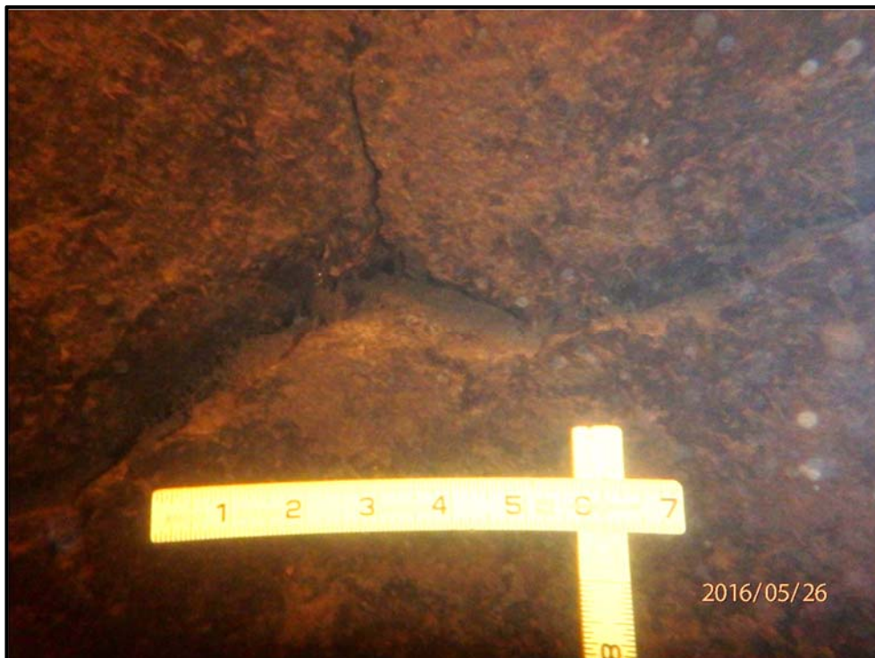
Photo 8 – Typical Horizontal Crack in Exposed Footing (Pier 2 Shown, East Nose)
