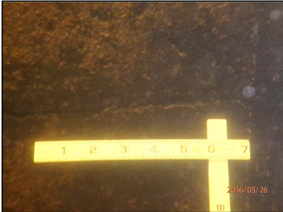
Photo 7 – Typical Horizontal Crack in Pier (Pier 4 Shown, West Face)
