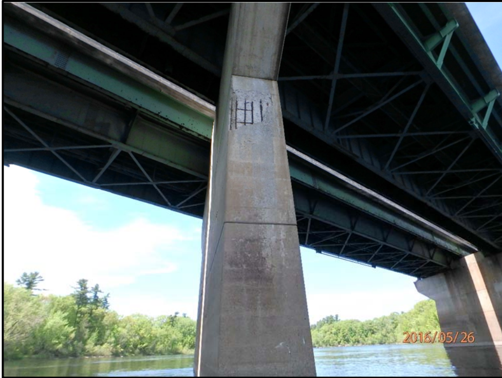
Photo 5 – Typical Spall with Exposed Reinforcing Steel (Pier 3 Shown, South Face)
