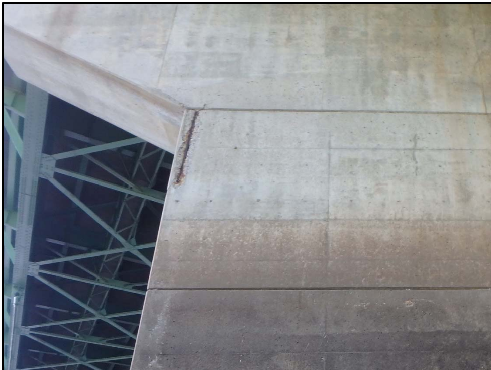
Photo 6 – Typical Spall with Exposed Reinforcing (Pier 4 Shown, East Face)
