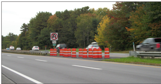
THE GUARDRAIL IMPROVEMENT PROGRAM HAS BEEN COMBINED WITH THE PAVEMENT REHABILITATION CONTRACTS
