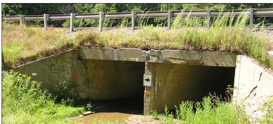
THE PISCATAQUA RIVER RELIEF CHANNEL, ORIGINALLY BUILT IN THE 1950'S, IS CURRENTLY UNDER REPAIR
