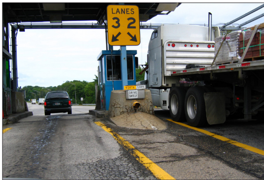
THE EXISTING YORK TOLL PLAZA HAS NUMEROUS DEFICIENCIES AND SAFETY CONCERNS
