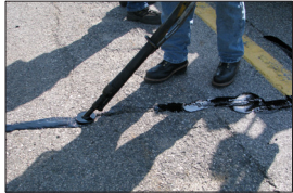
DISPENSED AT OVER 350 DEGREES, THE RUBBERIZED ASPHALT SEALANT IS INJECTED DIRECTLY INTO THE PAVEMENT CRACKS
