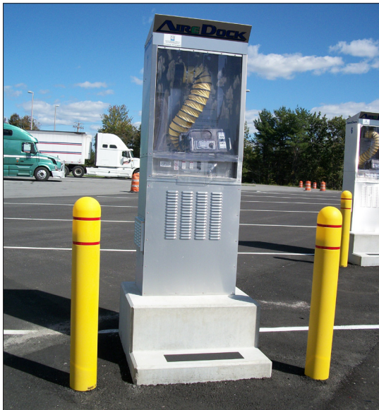
IN 2009 A TRUCK STOP ELECTRIFICATION (TSE) SYSTEM WAS INSTALLED AT THE GARDINER TRAVEL PLAZA
