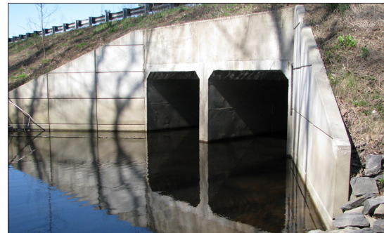
TWIN 8' X 8' CONCRETE BOX CULVERTS CARRY THACHER BROOK BENEATH THE MAINLINE IN KENNEBUNK
