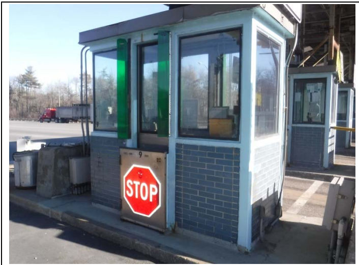
3. Typical brick "old" style toll booth – ACBM caulk, transite countertops and LP.
