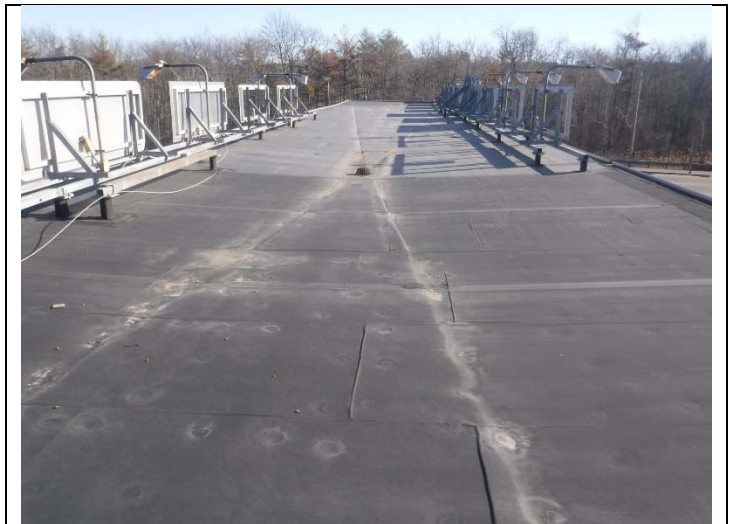
8. Canopy roof is EPDM rubber membrane on metal deck. No asbestos detected.
