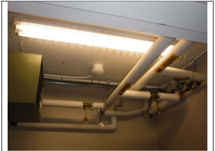
10. Piping throughout lower level of Administration Building is fiberglass. No suspect materials observed.
