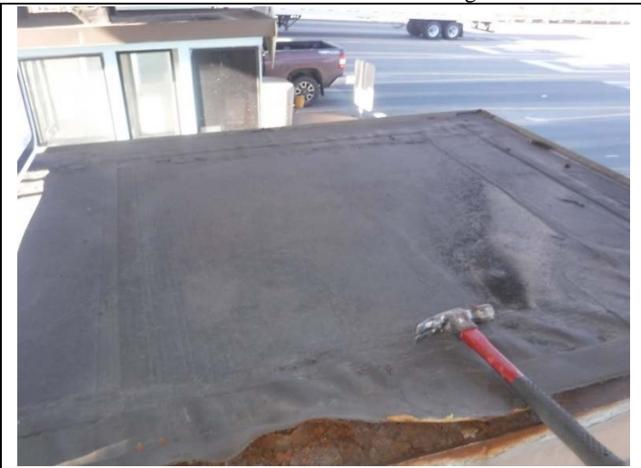
9. Brick style toll booths area EPDM rubber membrane roof on wood deck. No asbestos detected.
