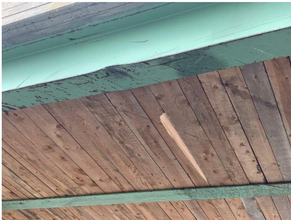
Photo 5 – Girder G1 Collision Damage (Looking North)
