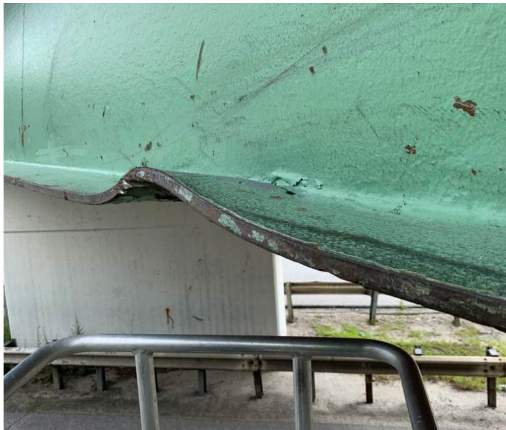
Photo 3 – Girder G4 Bottom Flange Deformation (Looking Northwest)
