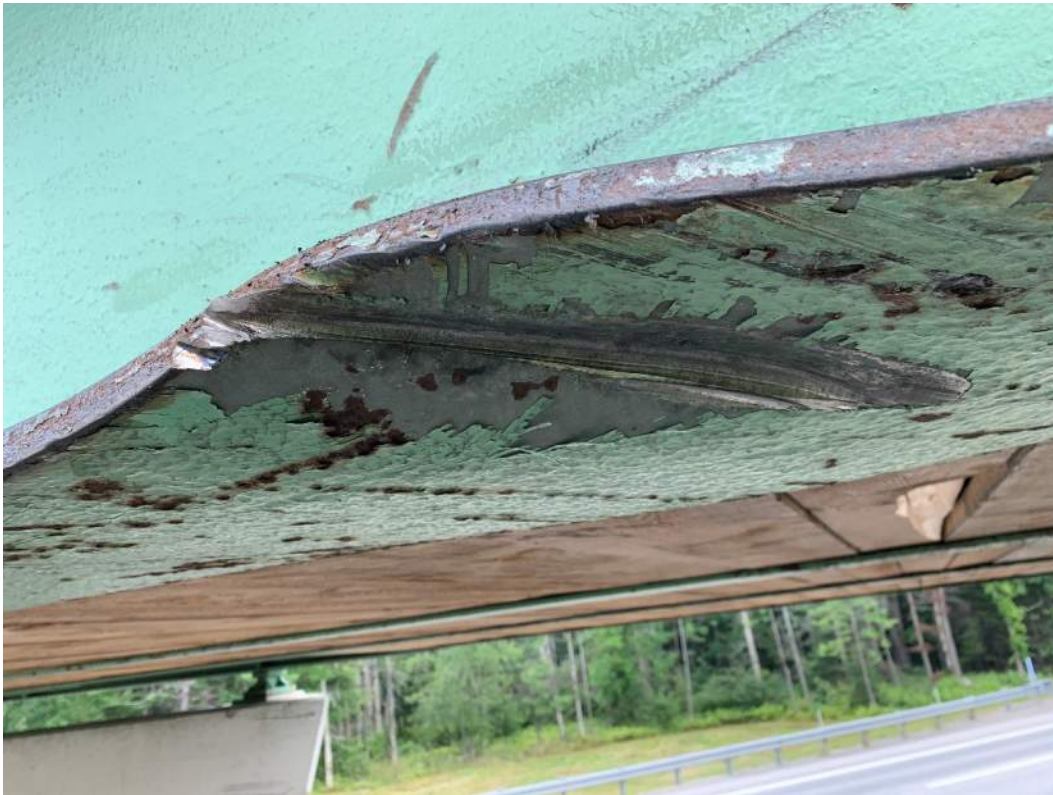
Photo 6 – Girder G4 Gouge and Deformation (Looking Northwest)
