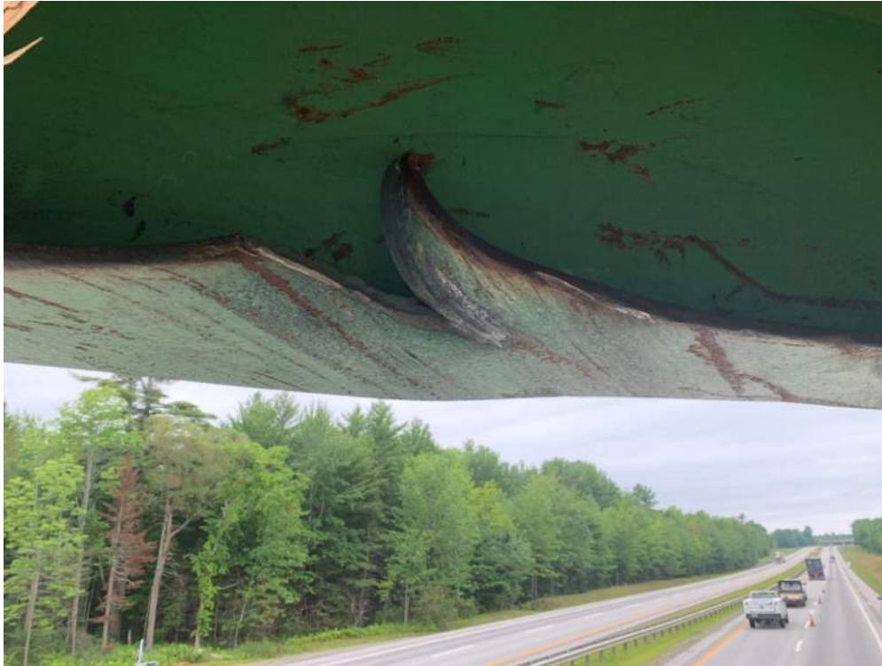
Photo 2 – Girder G4 Bottom Flange Tear (Looking South)
