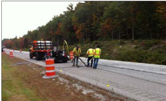
DISPENSED AT OVER 350 DEGREES THE RUBBERIZED ASPHALT SEALANT IS INJECTED DIRECTLY INTO THE PAVEMENT CRACKS
