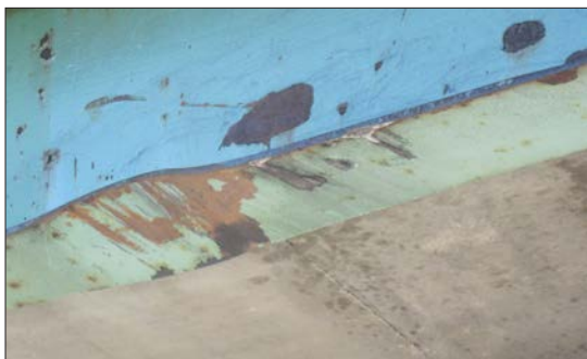
HACKETT ROAD UNDERPASS IMPACT DAMAGE, MILE 76.9
