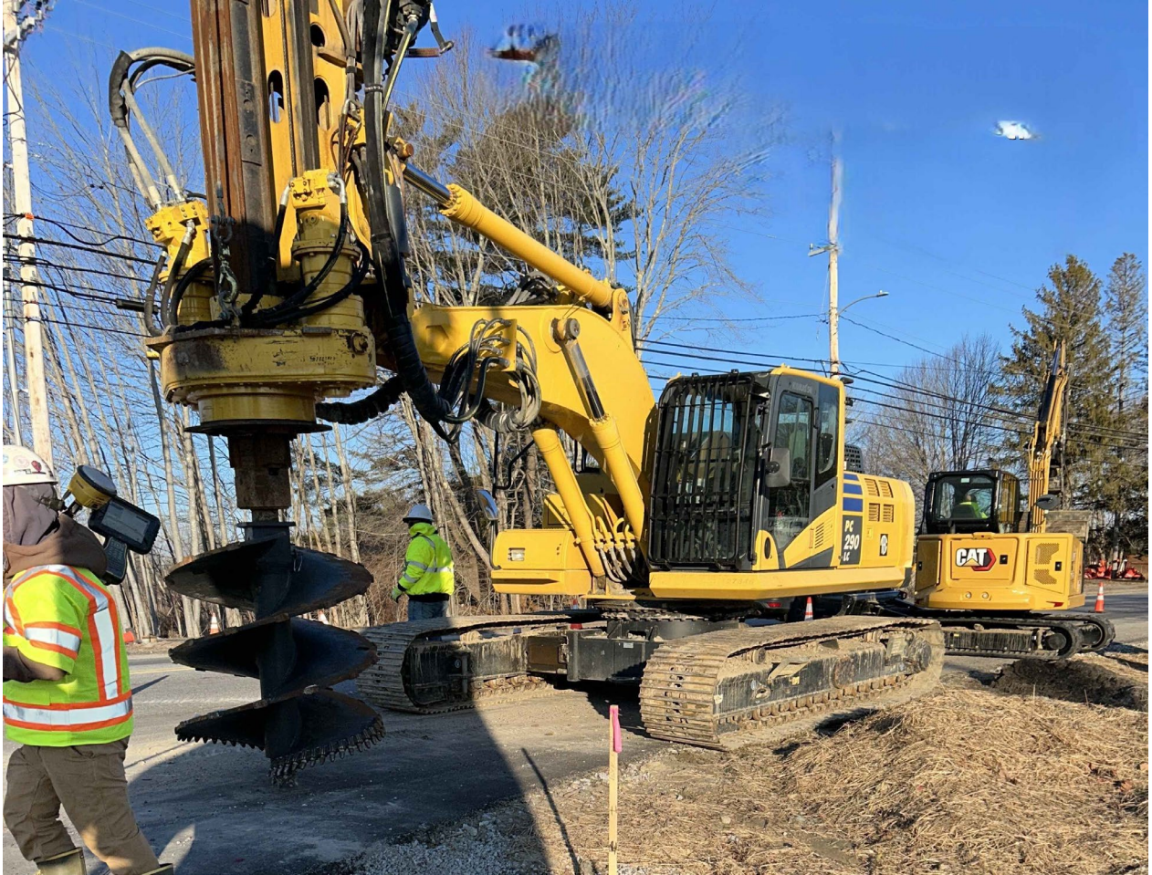
A sign foundation is about to be drilled at the Lund Road intersection
