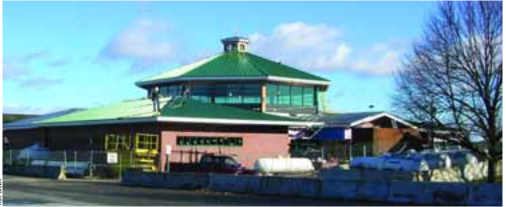
Construction began on new north and southbound service plazas at Kennebunk in the spring.
