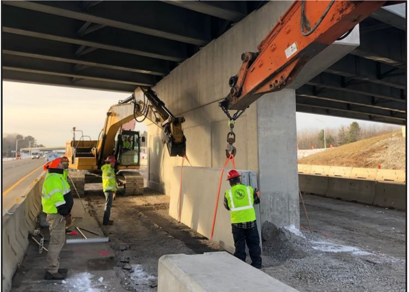
Looking north as a crew installs concrete barrier around the Exit 45 bridge pier.
