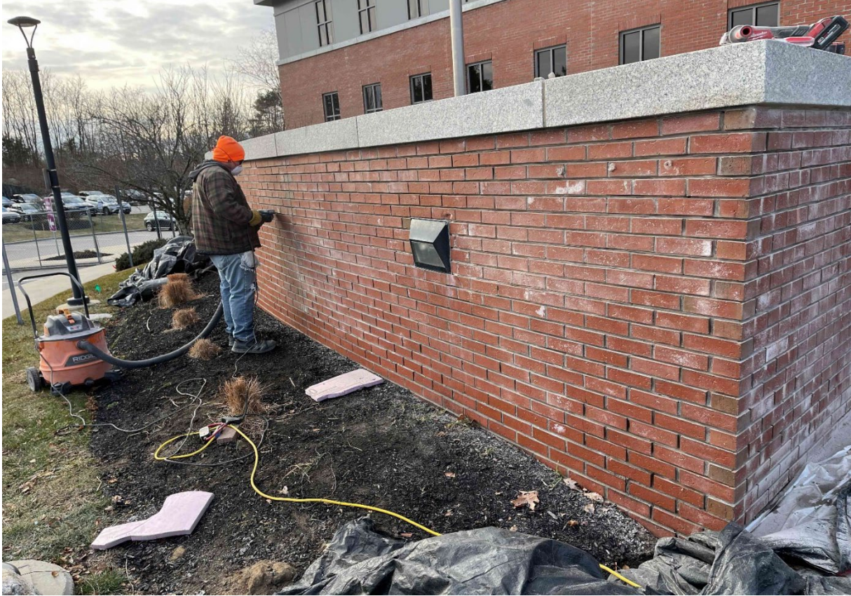
One of the masons is removing loose mortar from the brick work
