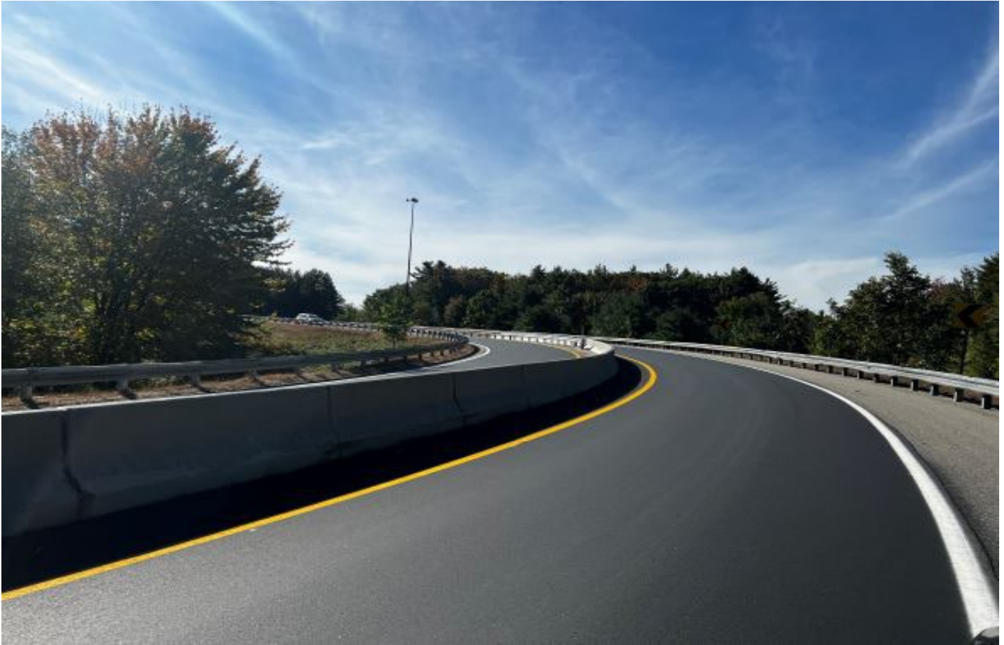
Exit 36 southbound exiting ramp, looking south, showing the recently paved and striped travel way.
