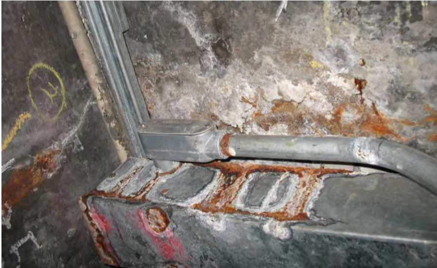
FIGURE 1.7 - Conduit Penetrations in York Tunnel
