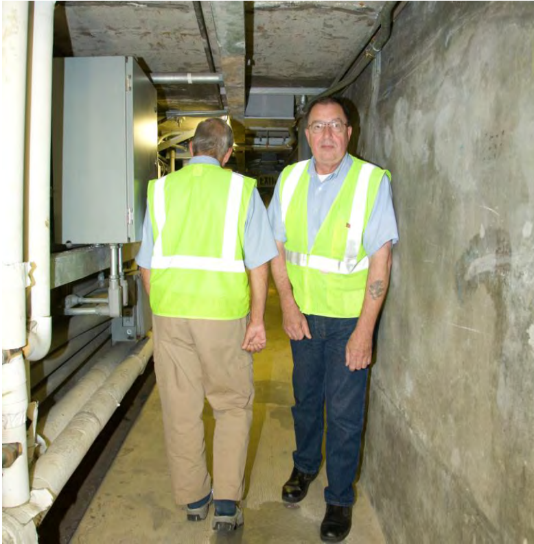
FIGURE 1.9 - York Tunnel Note, leak stains and narrow passageway.
