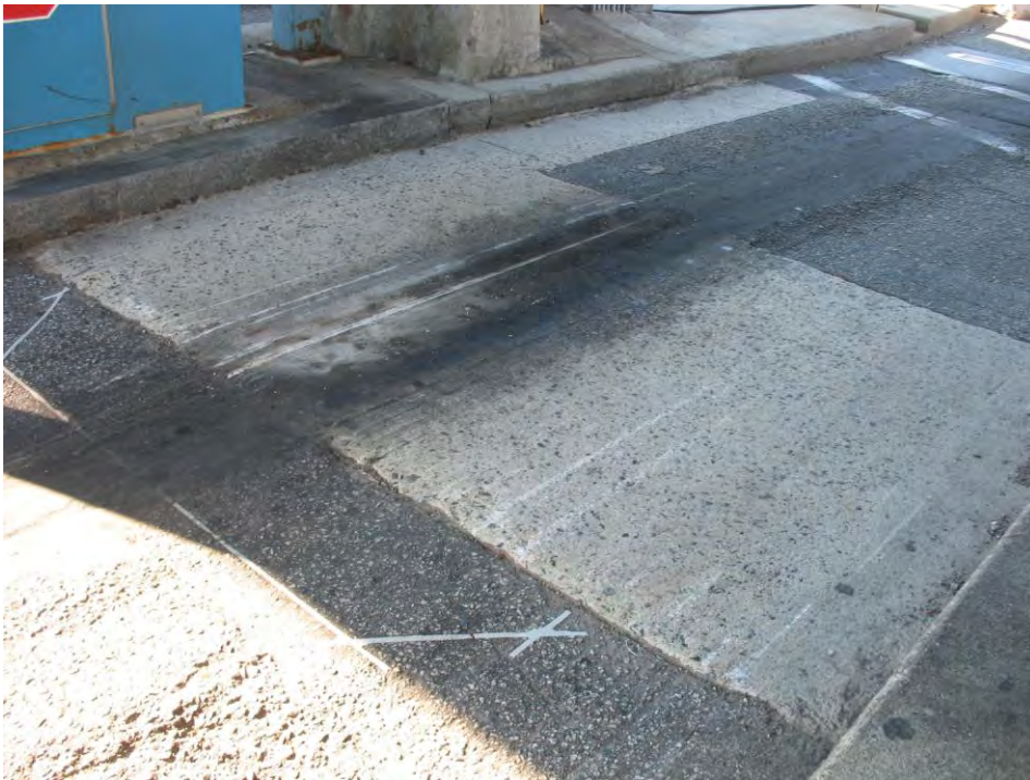
FIGURE 1.14 - Damaged Concrete Slab at Plaza
