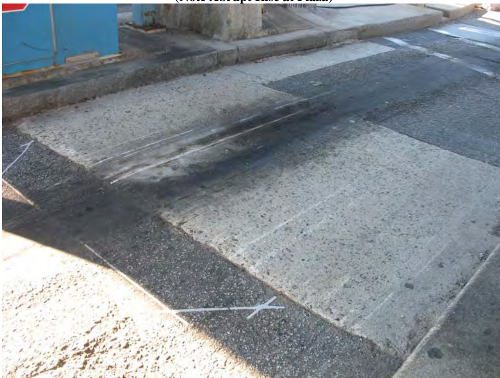
Figure 10 Damaged Concrete Slab at Plaza
