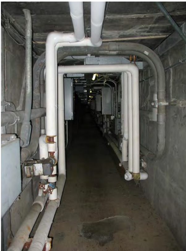
FIGURE 1.8 - Numerous Conduit Runs in York Tunnel
