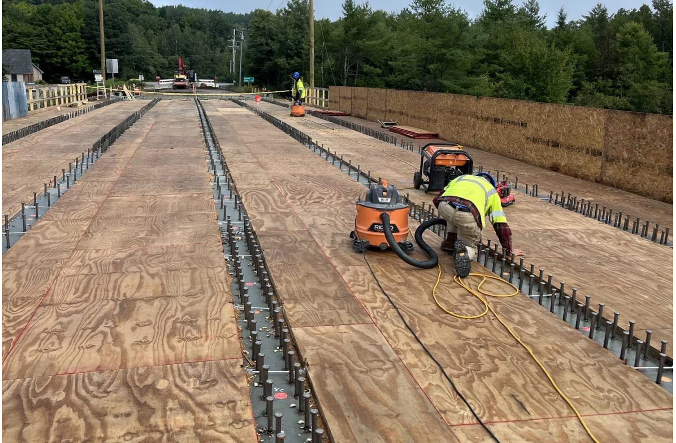
Looking west as crews clean the forms prior to placing reinforcing steel for the deck.
