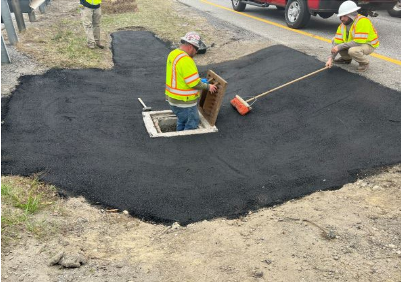
A crew is finishing repairs to a median catch basin in West Gardiner.
