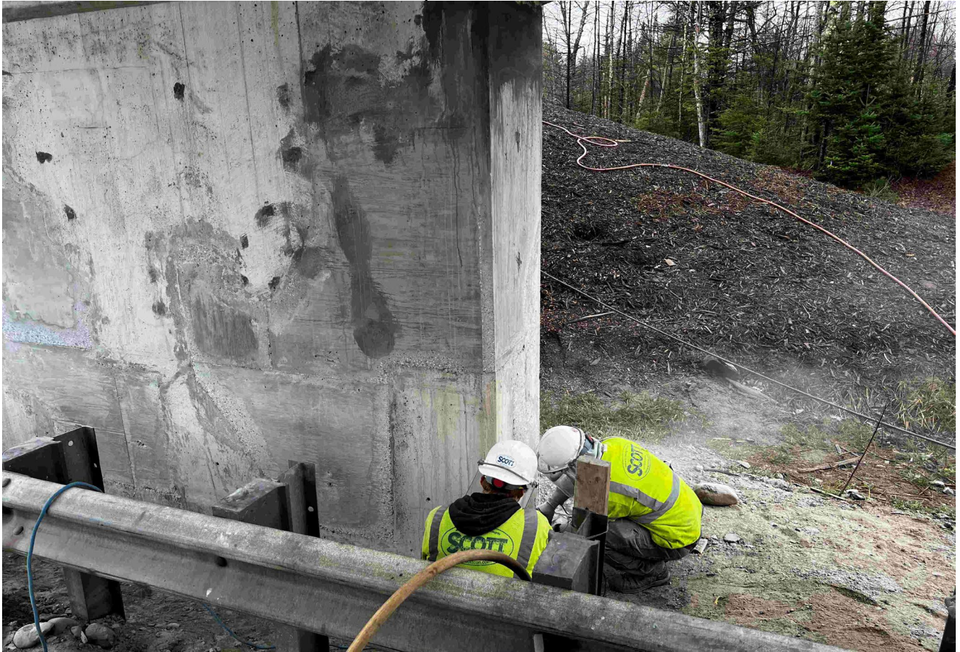
Looking at the northbound pier where crews are finishing up some concrete repairs.
