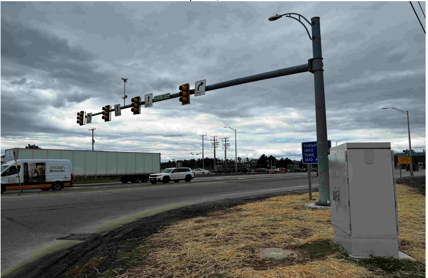
Looking west, the relocated mast arm, new foundation, and new controller cabinet for the Exit 42 intersection.
