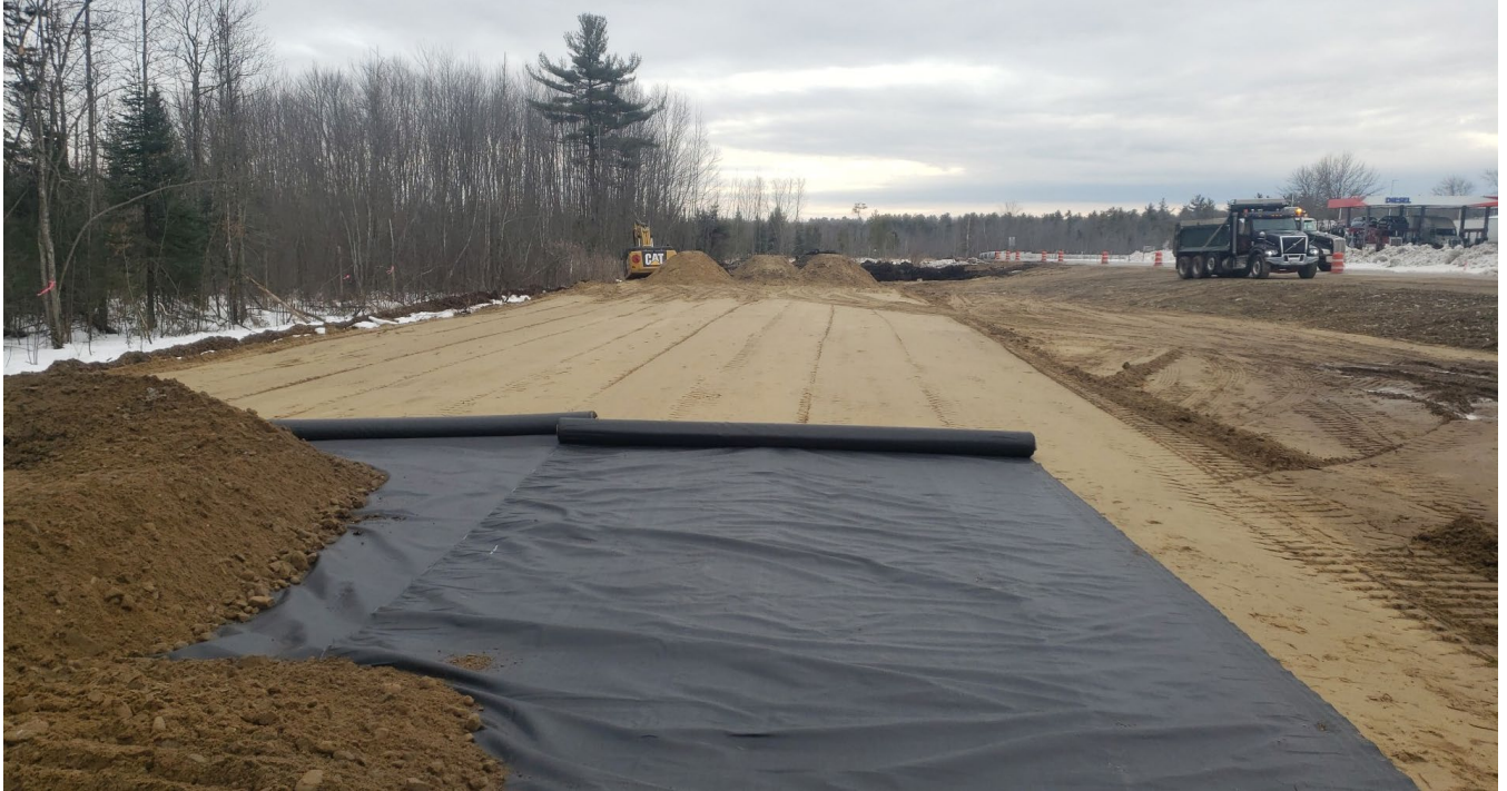
Subgrade and gravel layers of the relocated northbound on ramp, looking south.
