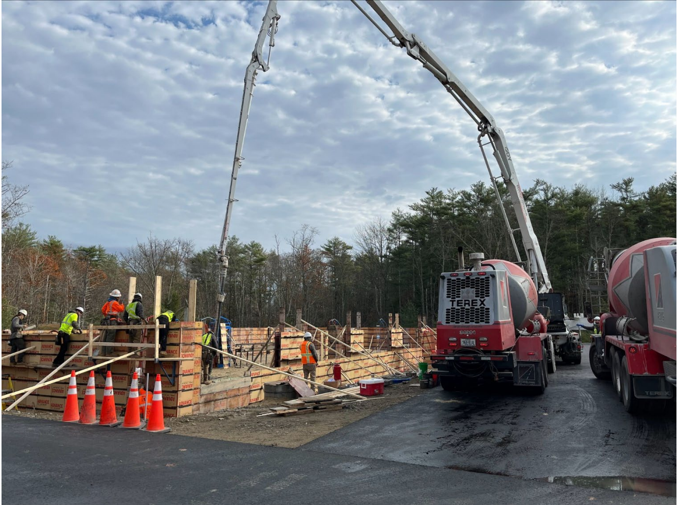
A concrete truck unloading into the pump used to fill the forms for the new foundation.
