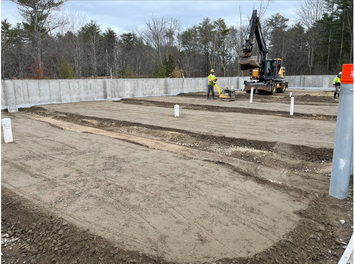
Earthwork crews backfilling the foundation around the drain lines and conduit runs.
