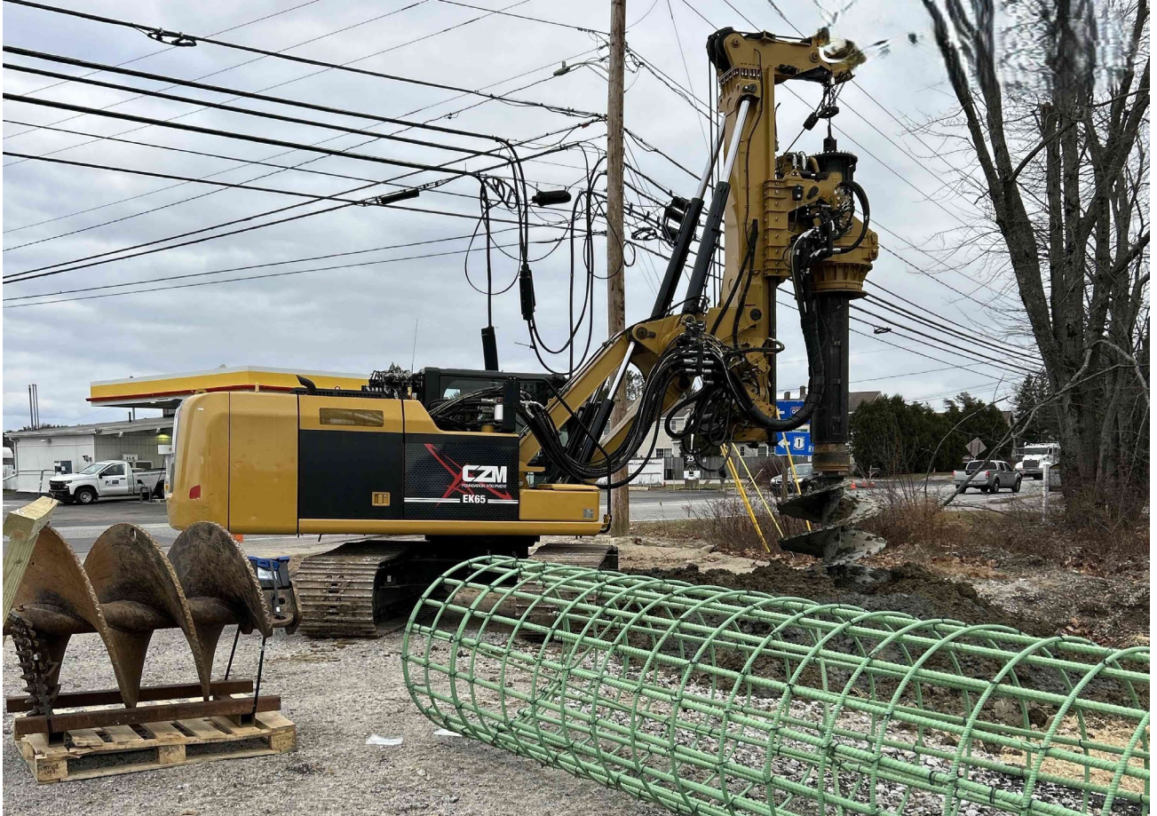
The contractor is augering for the signal mast foundation at the Route 112 northbound intersection
