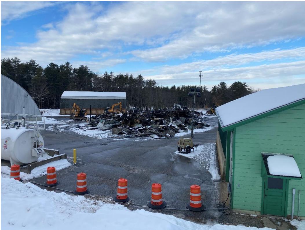
Photo 5 – Building remnants, including equipment
