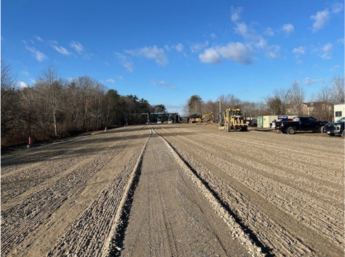
Sargent's grader is fine grading the northbound approach to Exit 35 from Route 112.
