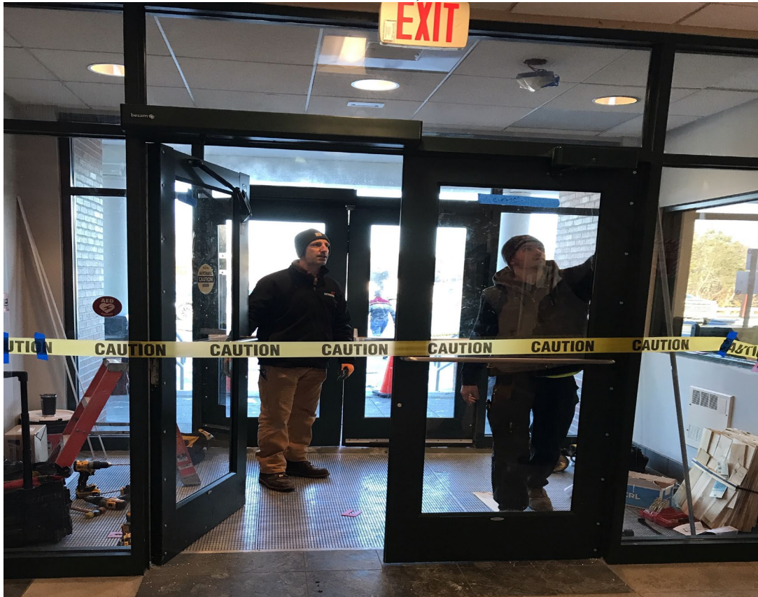
The front entrance to the Cumberland Service Plaza. Crews are installing the new doors.
