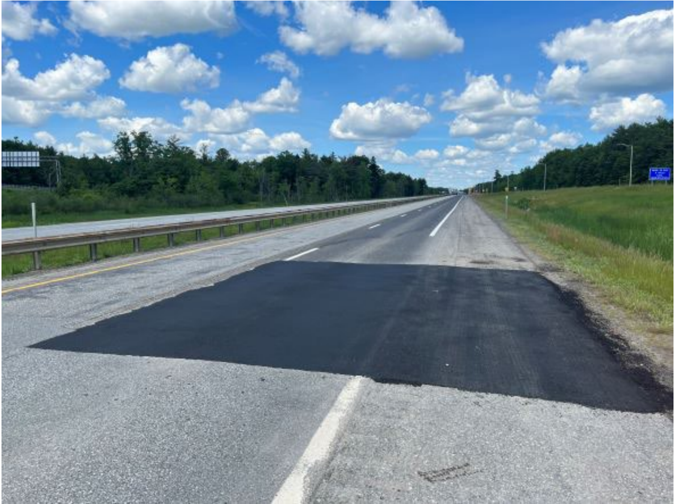
The start of the northbound milled area just south of the exit 103 entering ramp.
