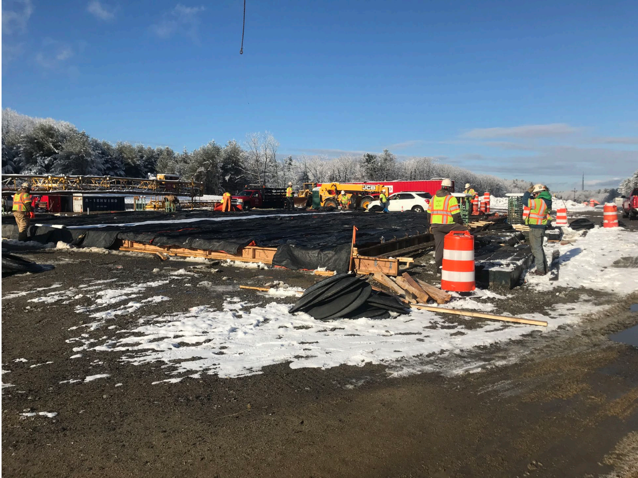
Reed & Reed employees removing exterior bracing from the northbound ORT concrete slab.
