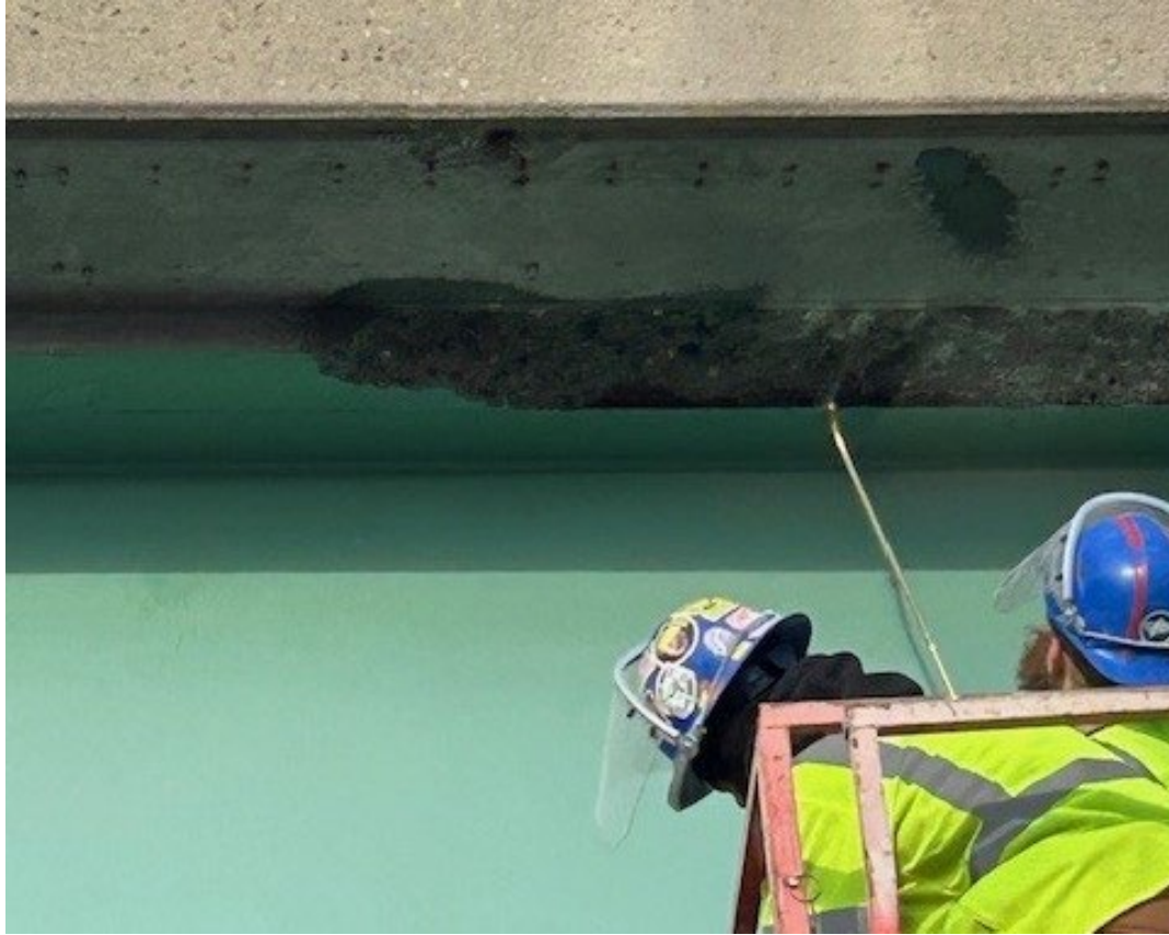
Cedar Hill Bridge showing a section recently removed concrete haunch.
