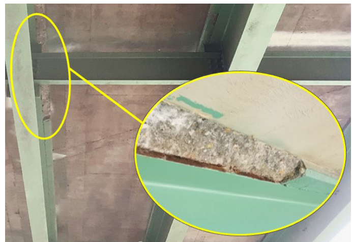
LEIGHTON ROAD UNREINFORCED HAUNCH SPALLS
