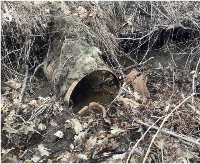
TYPICAL DETERIORATED PIPE/OUTLET
