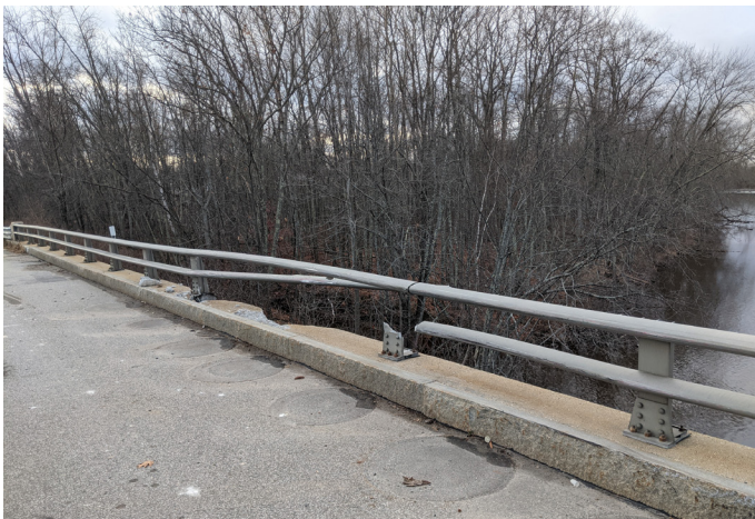
SACO RIVER OVERPASS DAMAGED BRIDGE RAIL
