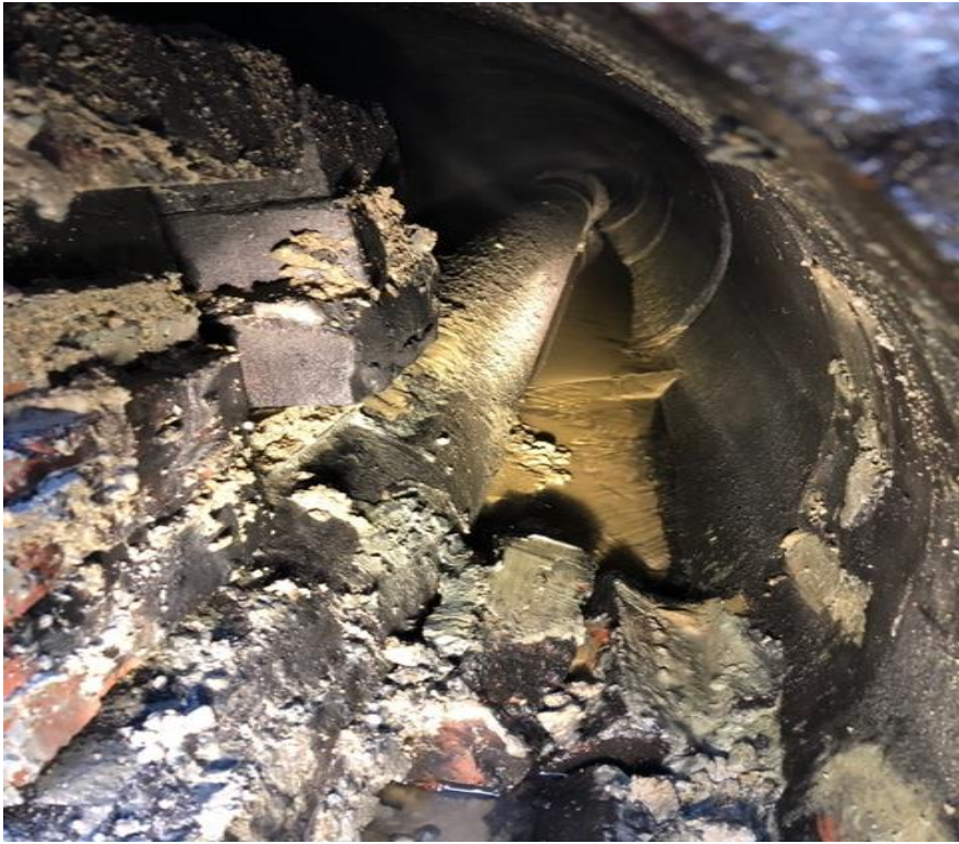
View From Casing End
