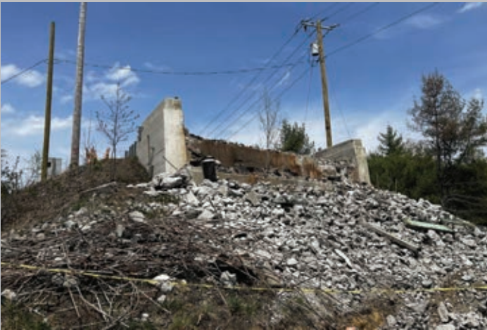
The remains of the old Route 122 Bridge in Auburn in May 2024
