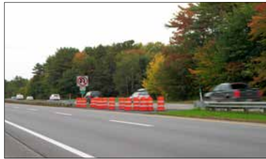
THE GUARDRAIL IMPROVEMENT PROGRAM HAS BEEN COMBINED WITH THE PAVEMENT REHABILITATION CONTRACTS
