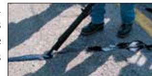
DISPENSED AT OVER 350 DEGREES THE RUBBERIZED ASPHALT SEALANT IS INJECTED DIRECTLY INTO THE PAVEMENT CRACKS
