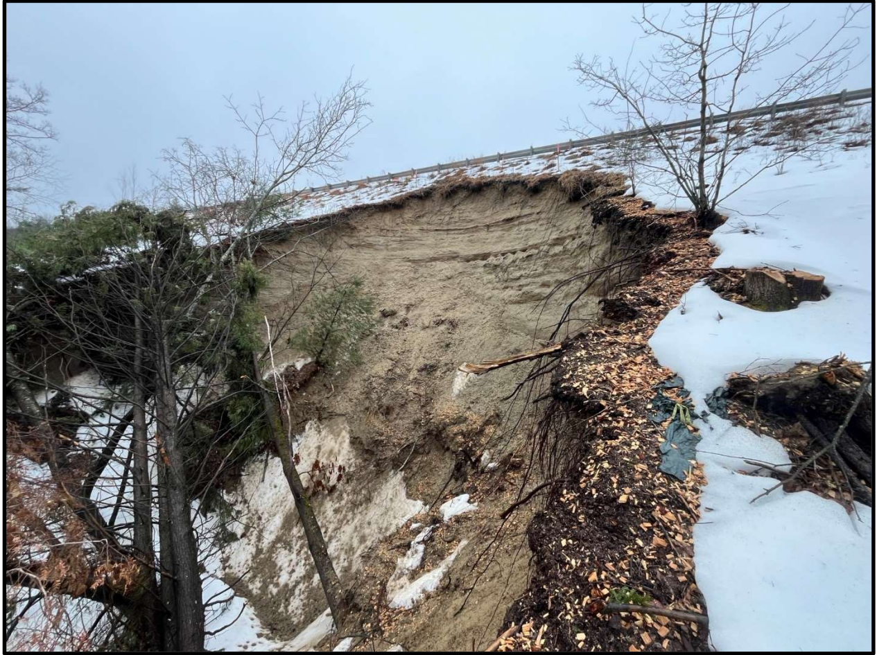
Figure 1 - Northbound Slope Failure before slope stabilization
