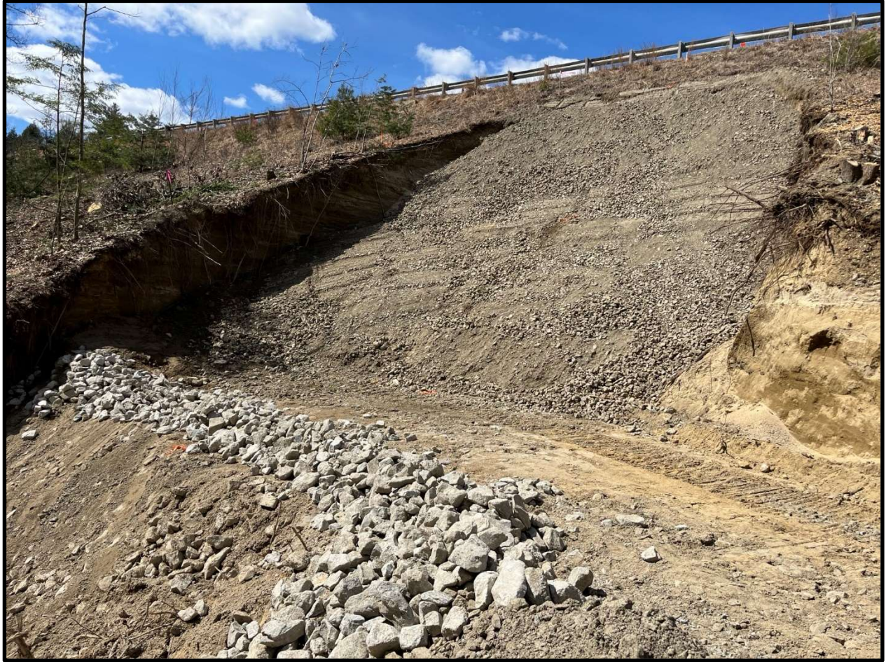
Figure 2 - Northbound Slope Failure stabilized with riprap, sand, erosion stone, and gravel backfill
