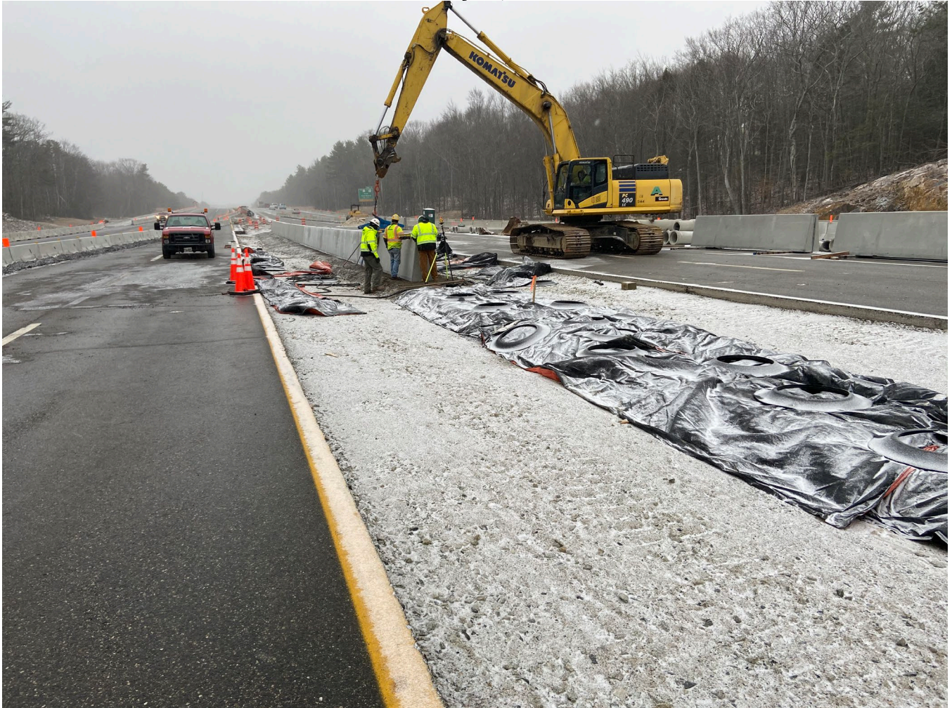
R.J. Grondin crew installs precast concrete median barrier south of the new ORT. (Looking south)
