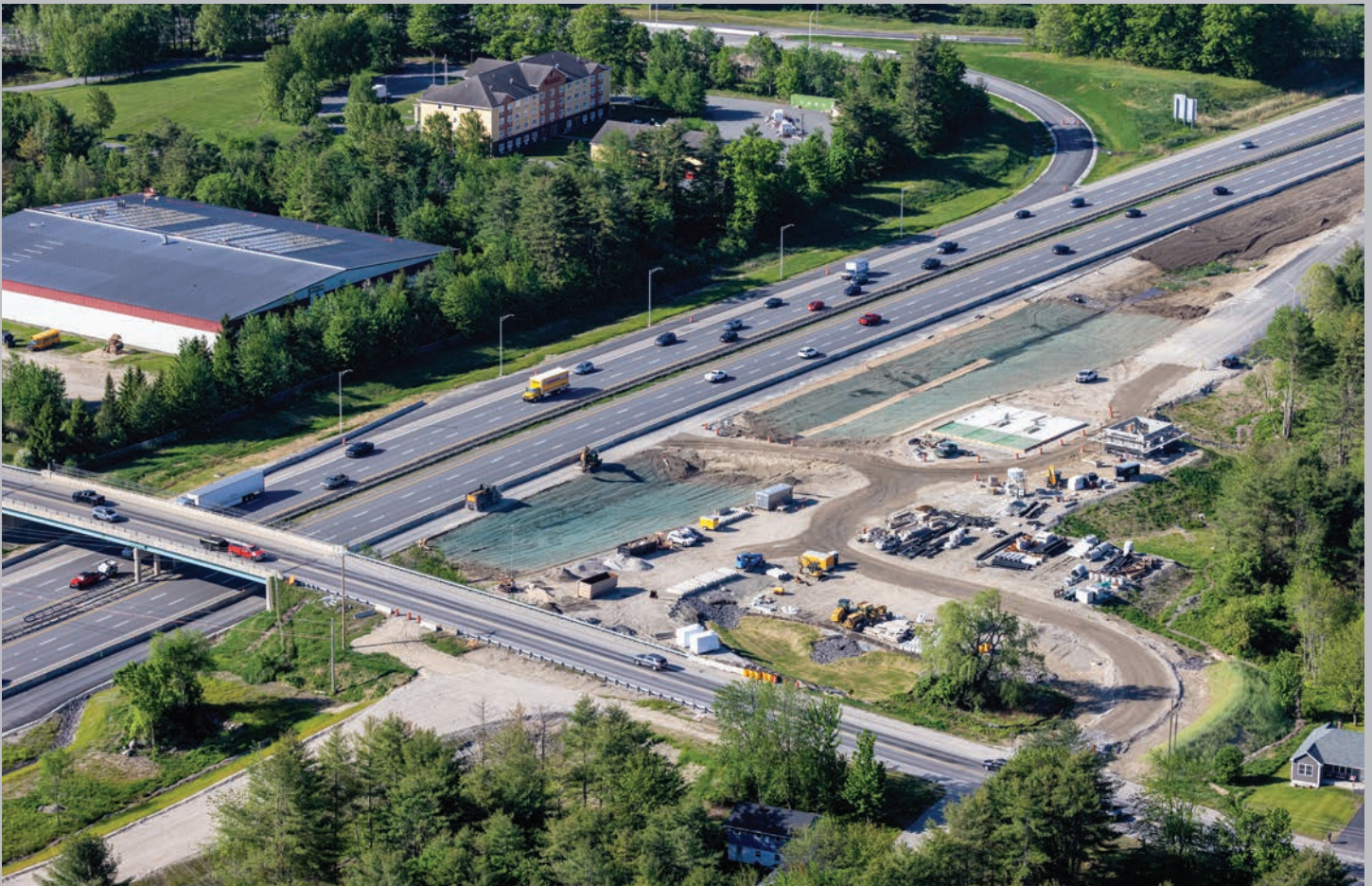
The new southbound on-ramp and toll plaza area at Exit 35 in Saco in May 2024.
