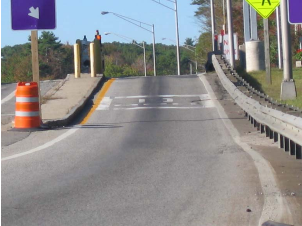
Figure 9 Settlement of Approach Slab (Note Abrupt Rise at Plaza)
