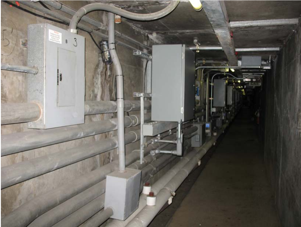
Figure 6 York Tunnel (Note Leak Stains and Narrow Passageway)
