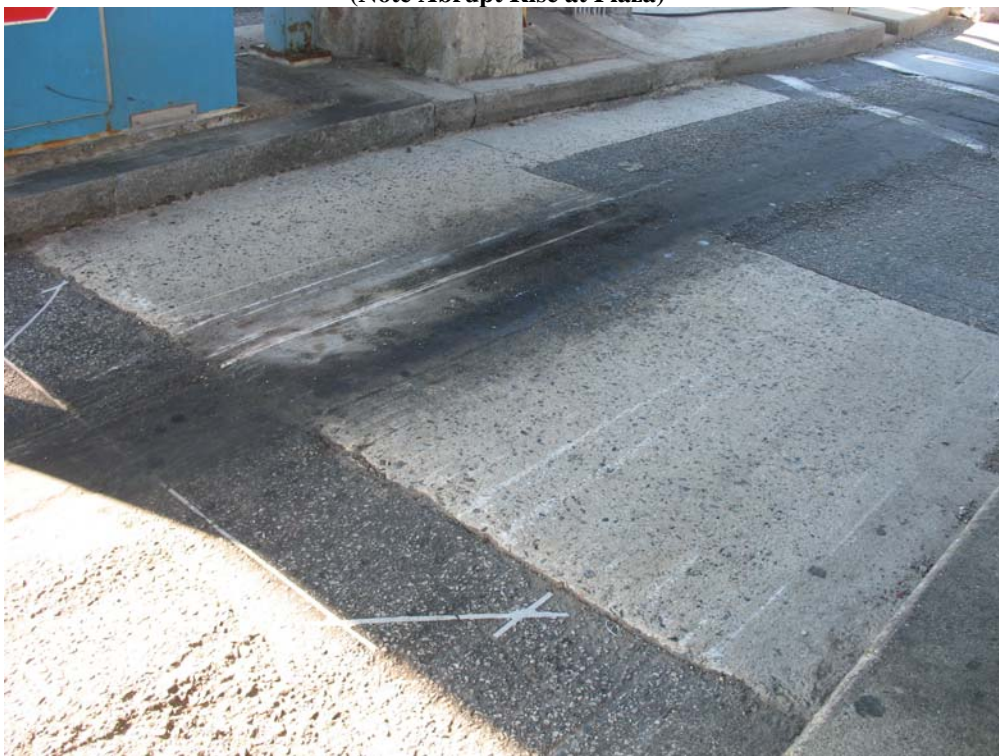
Figure 10 Damaged Concrete Slab at Plaza
