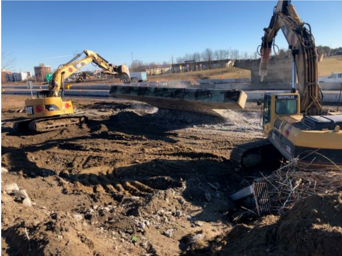
Looking east at the western bridge pier as it is knocked over by the contractor.
