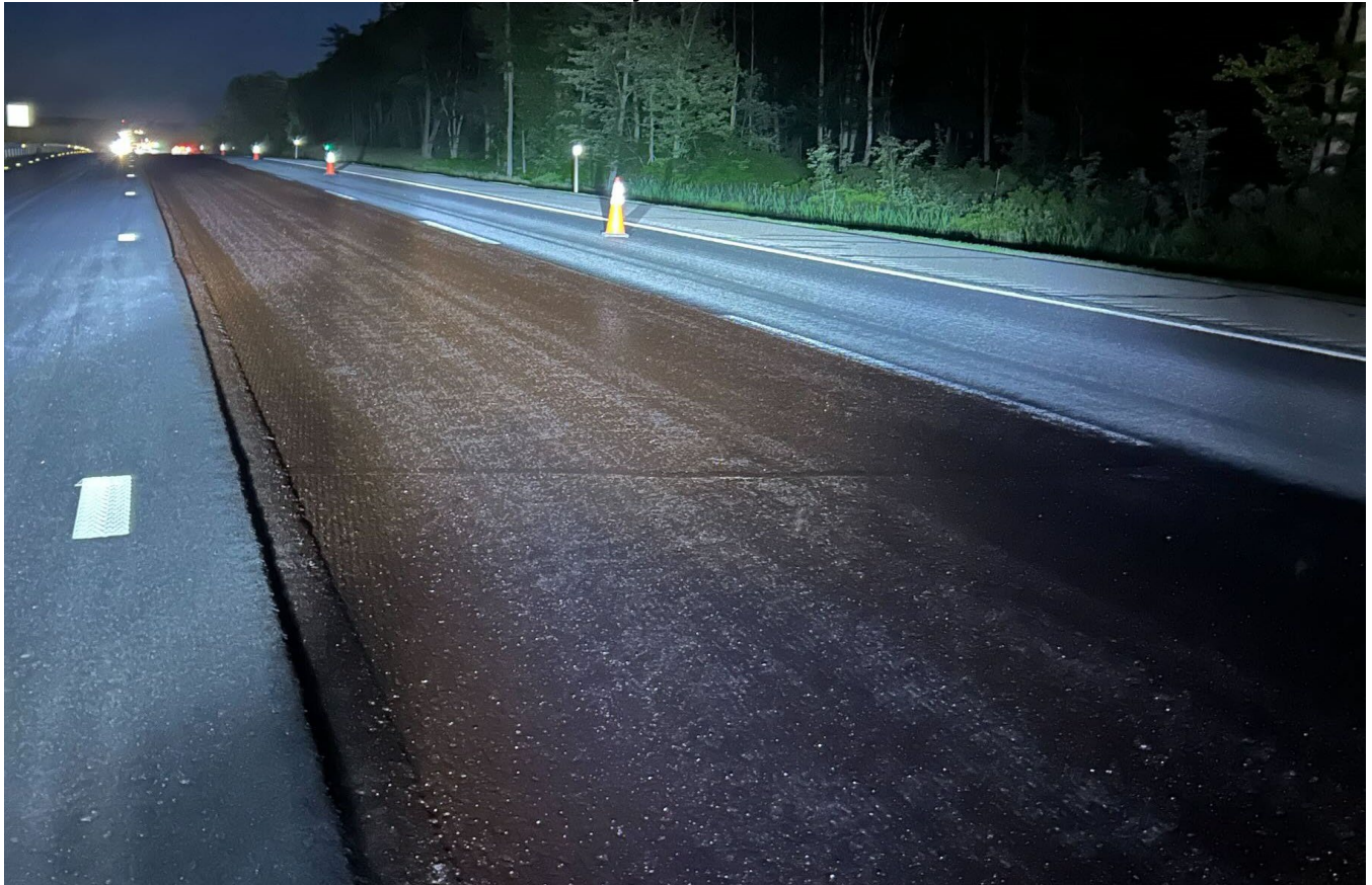
Southbound looking at lane 2 prior to being paved. The black liquid is tack that helps bond the pavement layers together.
